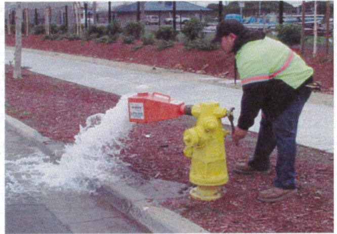
Our utility maintenance crew flushes a City fire hydrant. There are over 1,500 fire hydrants to maintain in the City.
