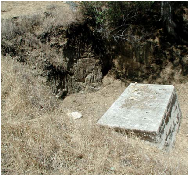
Above: Stamp mill foundation Patterson Mine, Millerton Lake State Recreation Area, SE ¼ Sect. 7, R22E T10S, elevation < 800' (would be inundated by MP 279 dam, and by MP 274 dam) (early afternoon). (P190084.JPG)
