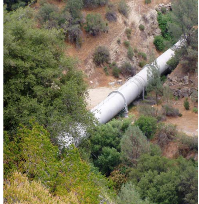
Above: Upper Redinger Lake, view east showing penstocks to SCE's Powerhouse 3 (mid-afternoon) (057.JPG)
