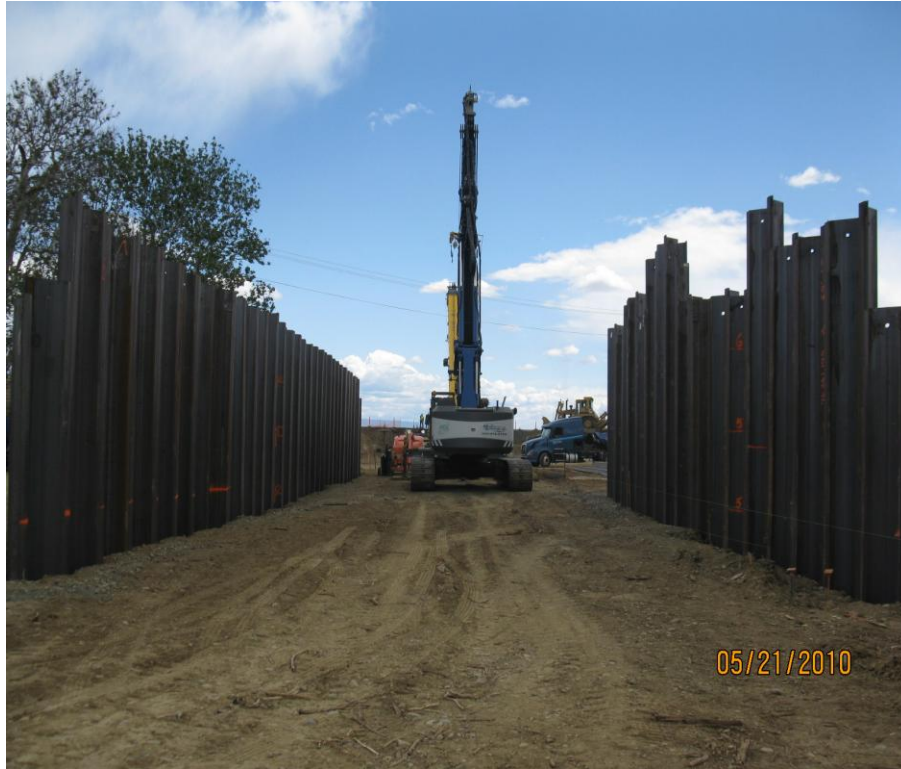
Sheet Piles for Canal on the East Side of Red Bank Creek.
