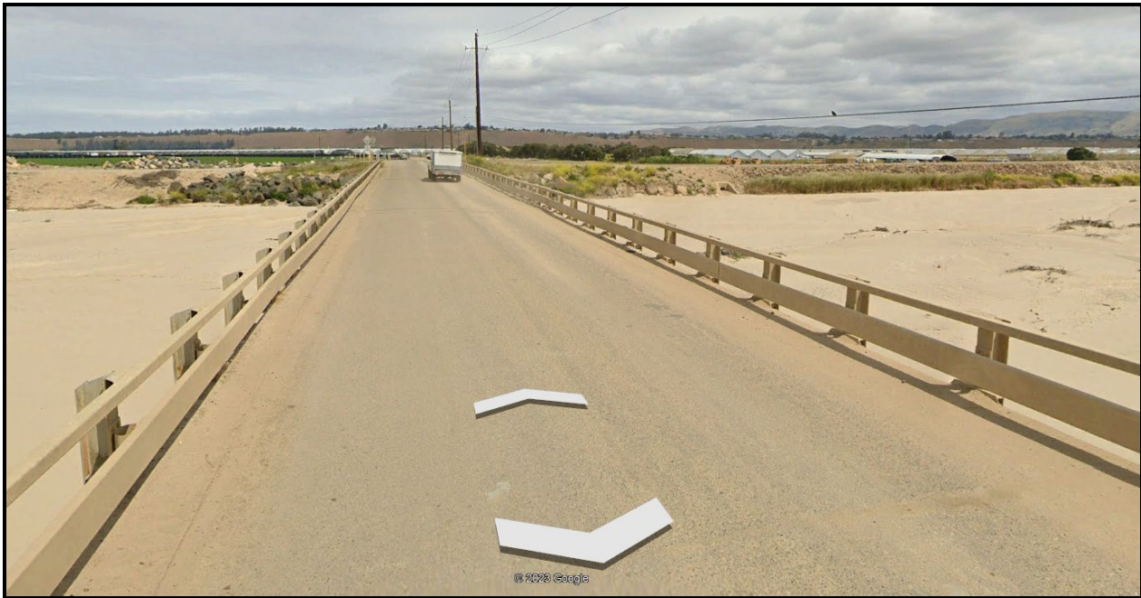
FIGURE 3: Bonita School Road Bridge. No walkway available
