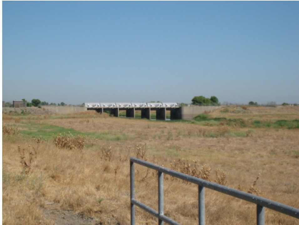
Figure 3.1-1. View of the Eastside Bypass Control Structure in Summer, Looking Downstream to the North
