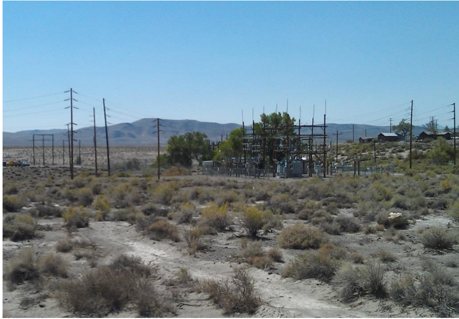
Figure 3. Existing Lahontan Substation
