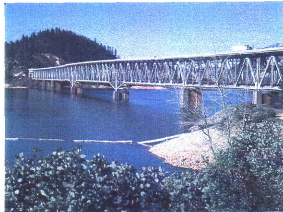
The Pit River Bridge, at Bridge Bay, carries vehicular traffic of Interstate 5 on its upper deck and railroad traffic on its lower deck. Piers 3 and 4, seen here in the center-left of the photo, where the truss superstructure dips down, govern the extent Shasta Dam can be raised without replacing the bridge.
