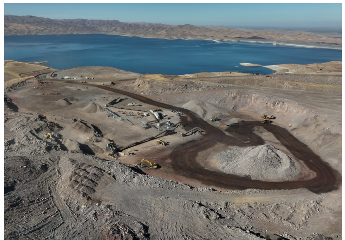
Construction is underway to improve the seismic reliability of B.F. Sisk Dam; it is Reclamation's largest project under the 1978 Dam Safety Act.
