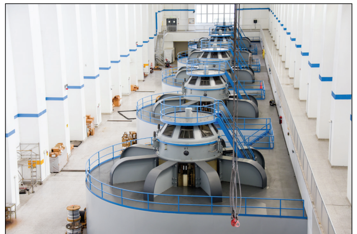
Five power generators operate inside of the Shasta Powerplant.
