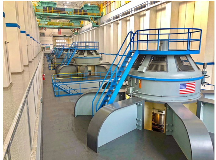
Five Shasta Dam hydropower pumps
