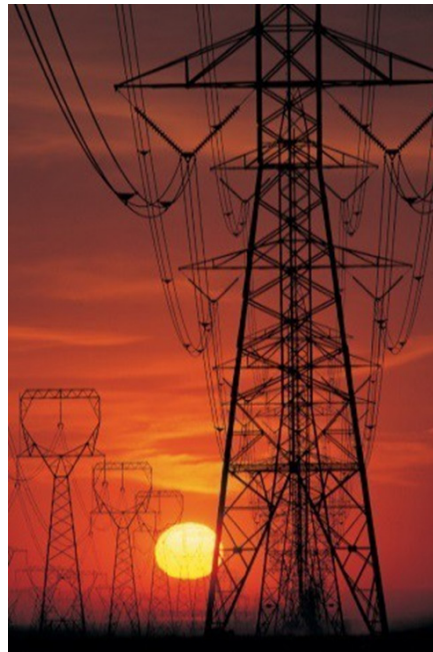
Powerlines transmitting hydropower.
