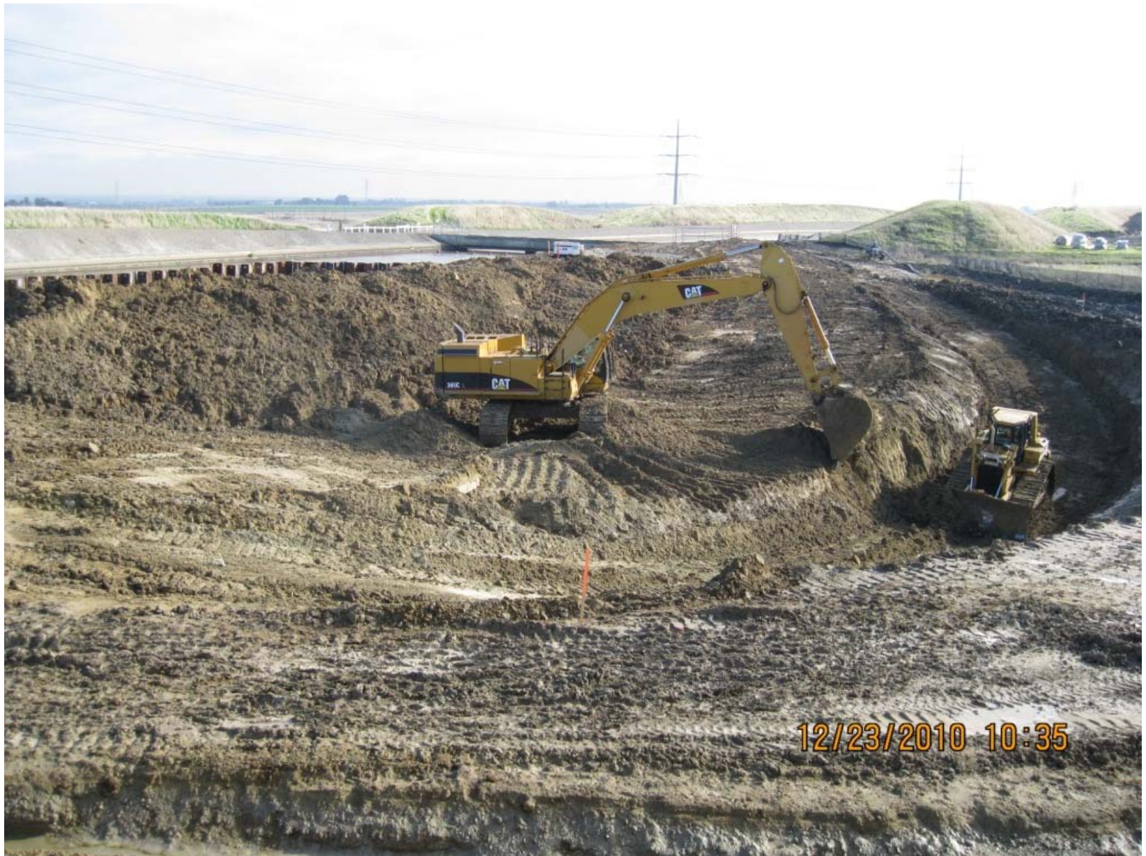
Mass Excavation of Pump Plant Structure working around rain and wet conditions
