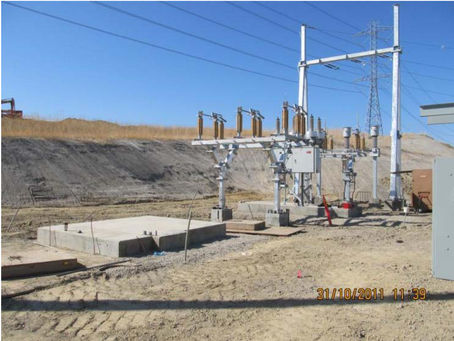
Switchyard transformer and circuit breaker concrete pads
