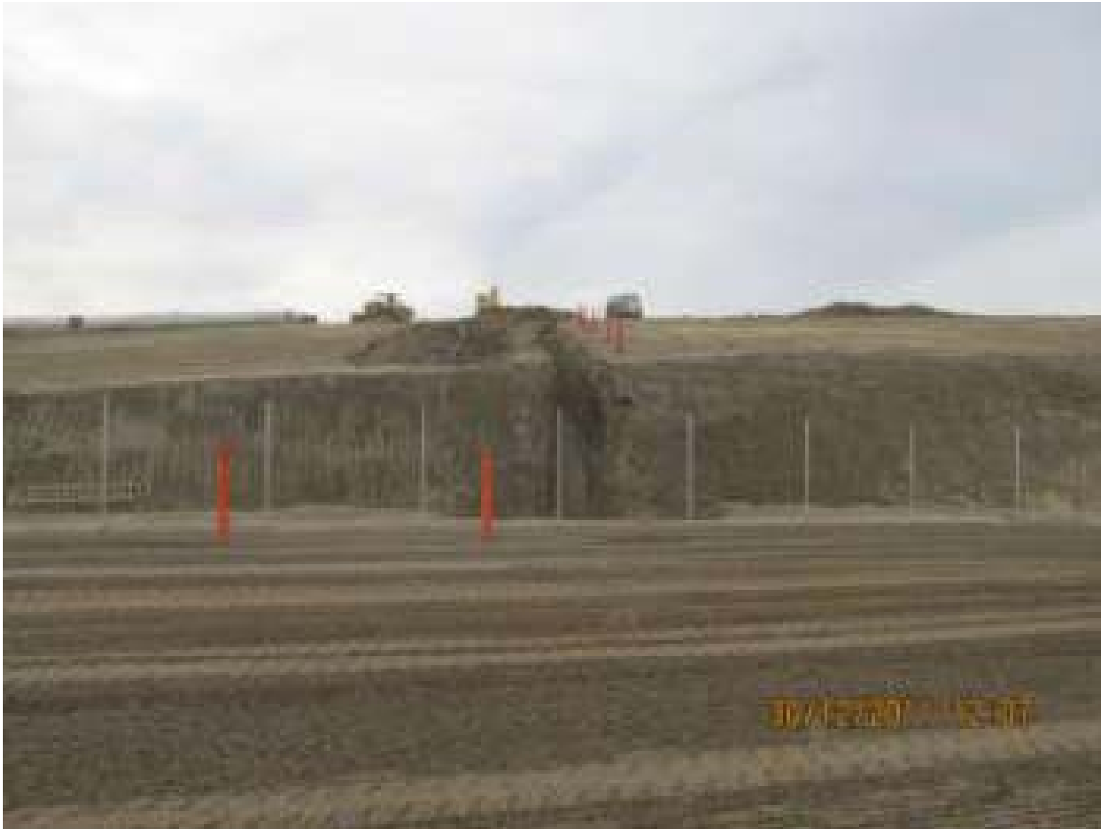
service yard and line pipe, December 30th. The orange posts at right are cathodic protection test stations.
