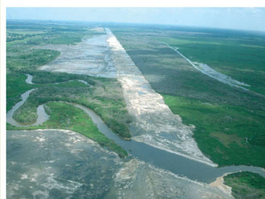
February 9, 2001, photo of implemented phase one Kissimmee River Restoration Project showing the backfilled canal, degraded soil area, remnant river channel, the connector channel, and wetland areas.
