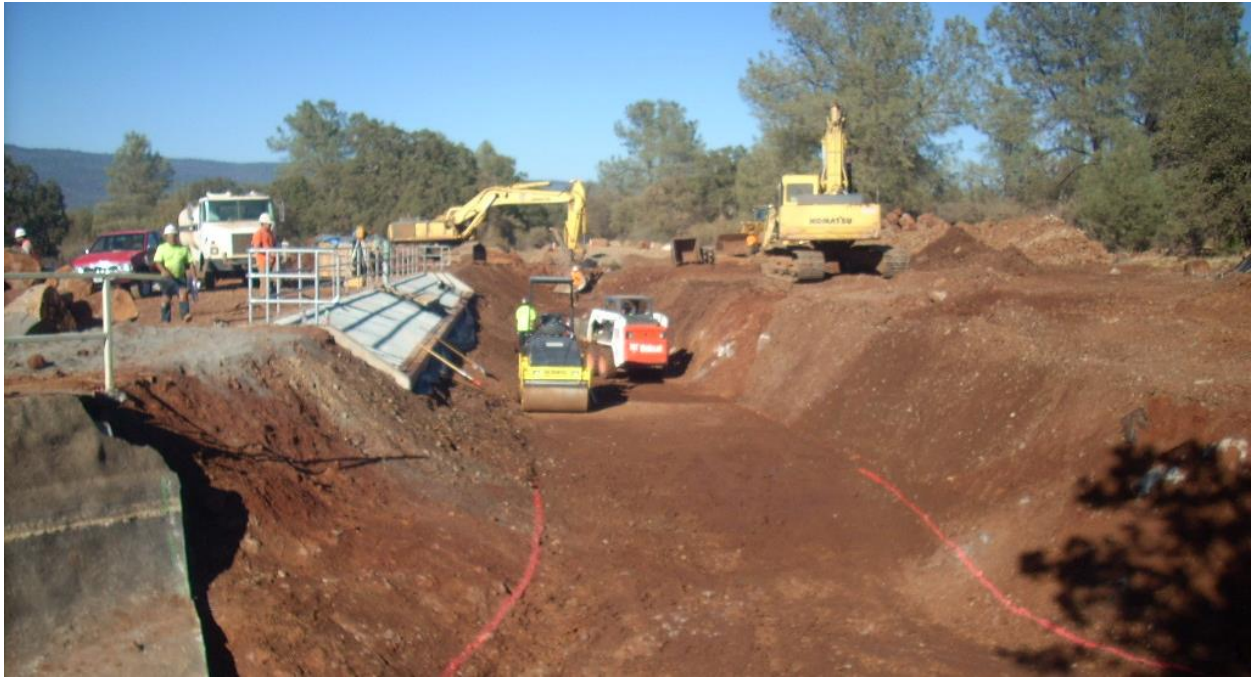
During construction photo looking upstream of Eagle Canyon Canal at the new Inskip Powerhouse penstock bypass intake structure (center left), August 2012.
