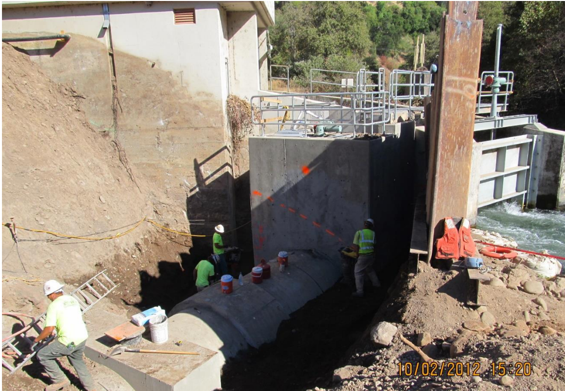
During construction photo of the new Inskip Powerhouse tailrace connector inlet structure (center) and the 84-inch buried pipeline (center bottom), October 2012.
