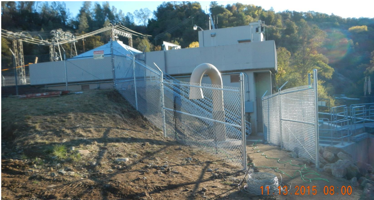
After construction photo of the new Inskip Powerhouse tailrace connector inlet structure (center right) and the 84-inch buried pipeline, November 2015.
