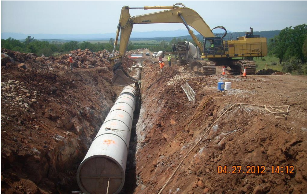
During construction photo of the Inskip Powerhouse penstock bypass, the 66-inch diameter buried concrete pipeline section, April 2012.
