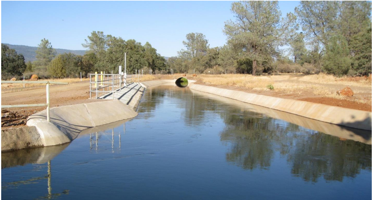
After construction photo looking upstream of Eagle Canyon Canal at the new Inskip Powerhouse penstock bypass intake structure (center left), September 2016.
