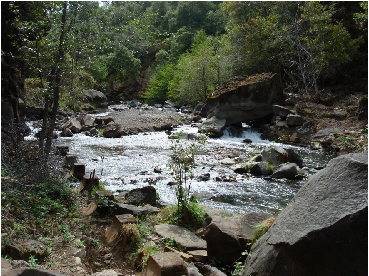
After construction, photo of North Fork Battle Creek immediately after the dam and pipeline were removed, September 2009.
