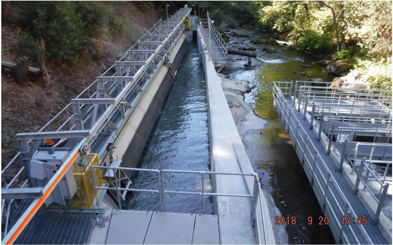
After construction, looking downstream at the new North Battle Creek Feeder pool and chute fish ladder (right) and the new diversion structure with fish screen (left), September 2018.
