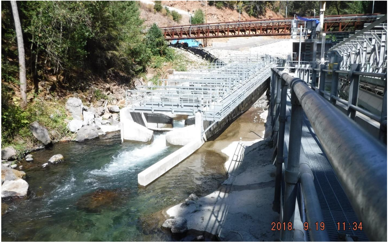
After construction, looking upstream at the new North Battle Creek Feeder pool and chute fish ladder (center) and the new screened diversion structure (right), September 2018.
