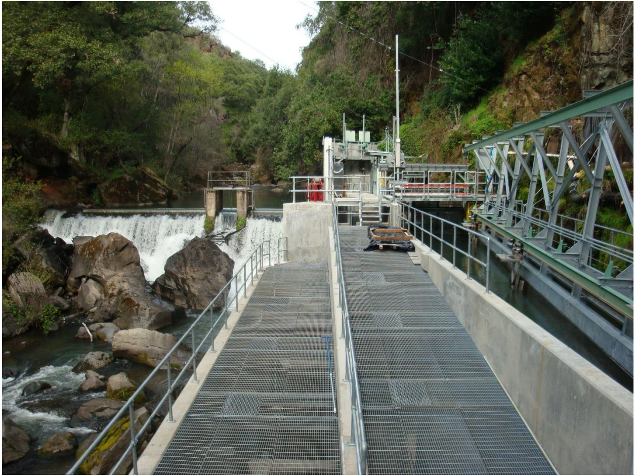
After construction, looking upstream at the new Eagle Canyon vertical slot fish ladder (center) and the new fish screen (right), April 2012.
