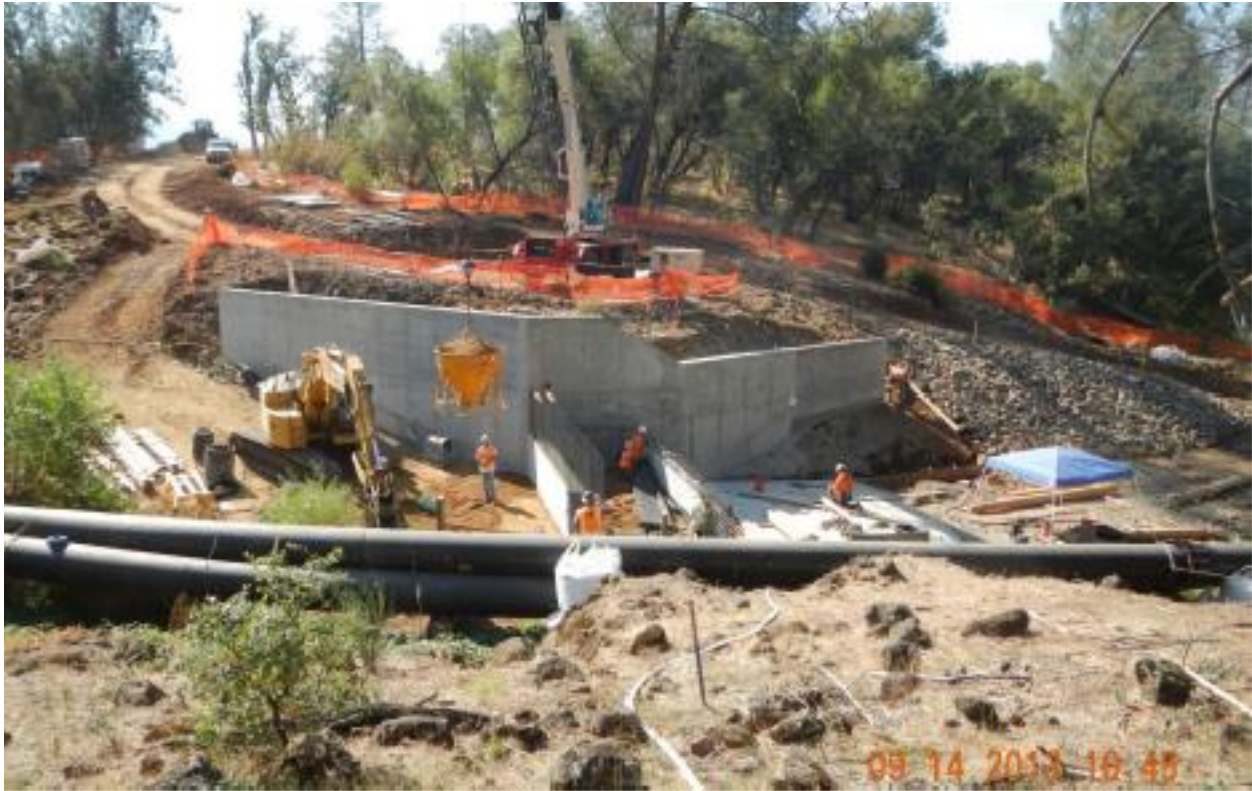
During construction, photo of the new Baldwin Creek fish barrier weir from the right bank, August 2013. The structure is located 500 feet downstream of Asbury Diversion Dam and Pump Station.
