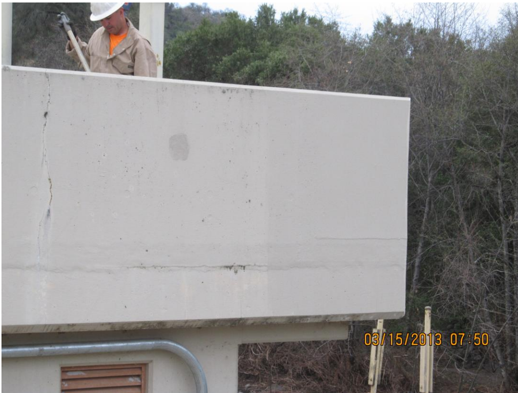
Coleman Diversion Dam/Inskip Powerhouse: The contract is finishing the final coating of the powerhouse parapet wall repair.
