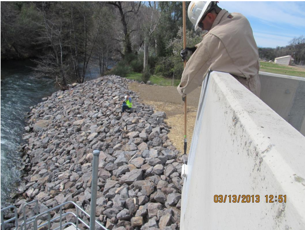
Coleman Diversion Dam/Inskip Powerhouse: Contractor RTA is applying primer coat follow by two coats of BASF Thorocoat elastomeric coating for the parapet wall repair.
