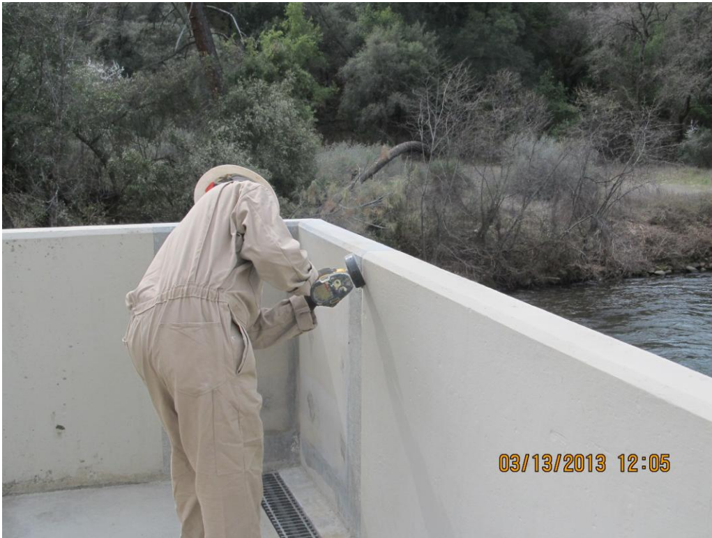
Coleman Diversion Dam/Inskip Powerhouse: The contractor is feathering existing coating for contact of new coating for the powerhouse parapet wall repair.
