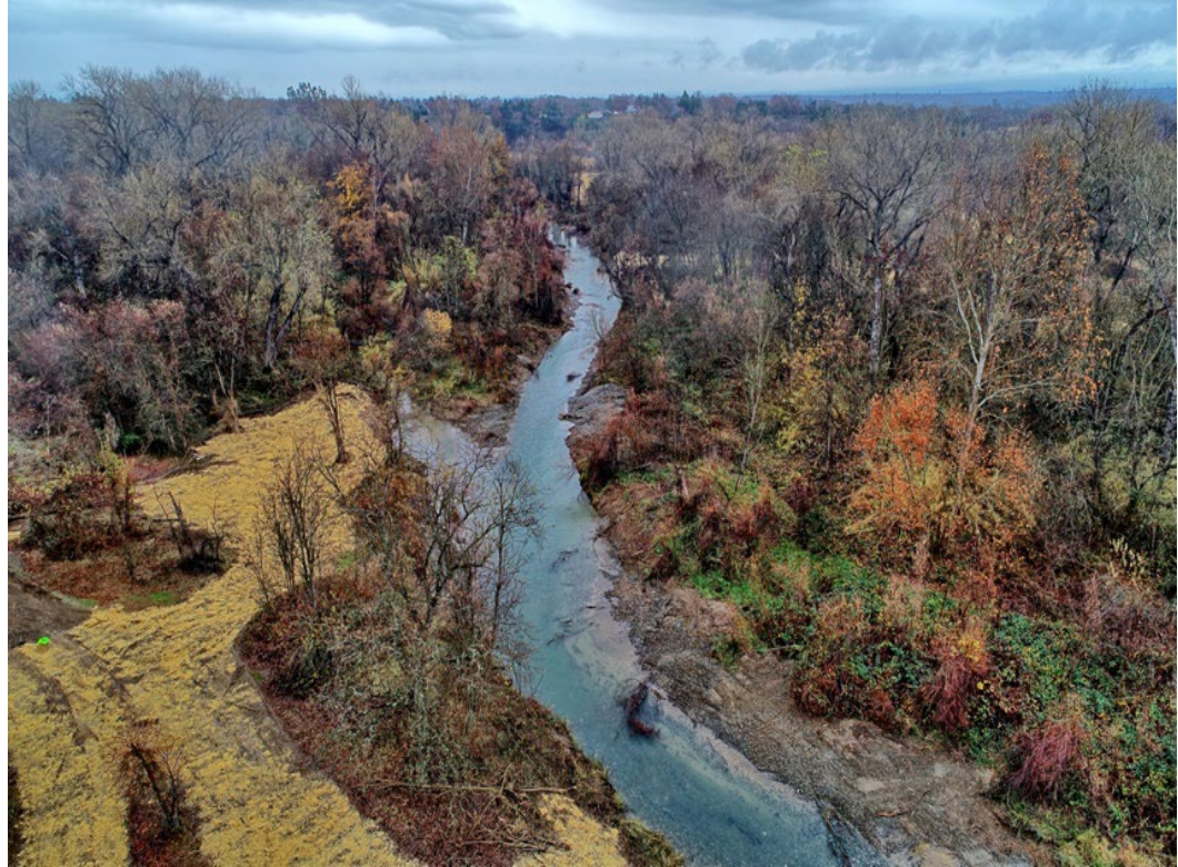
Anderson River Park Phase 1 Project after the side channel was excavated and reconnected to the Sacramento River, creating nearly one mile of new flowing salmonid habitat.
