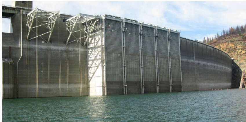
Photo showing Shasta Dam Temperature Control Device (TCD). The TCD allows colder water to be drawn from Shasta Reservoir and run through the generators. The water is then released into the Sacramento River to meet environmental needs for downstream fisheries.
