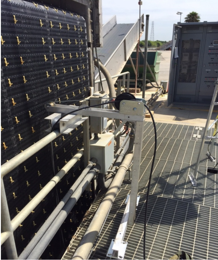
Figure 7. Photograph of Hydrolox screen panel No. 1 with yellow debris pegs. The velocity probe winch and trolley system is shown in the foreground. The conveyor debris collection system is shown in the background.
