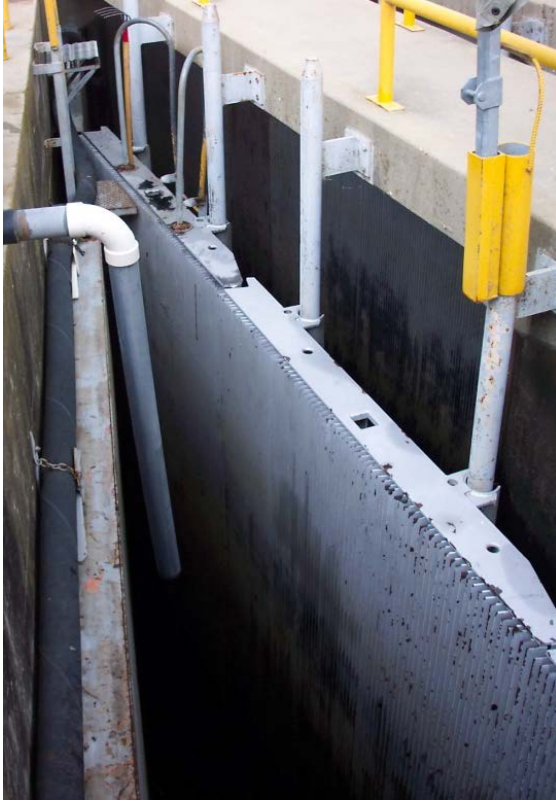
Figure 2. Original louver system in secondary channel.
