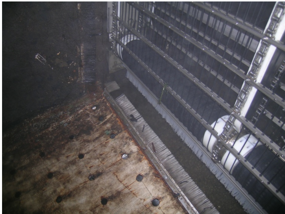
Figure 2c.—Vertical traveling screen 30.5 cm off the secondary channel, floor-steel plate inclined 33.0 cm (crab condition). Note 7.6 cm gap between 2 sets of brushes.
