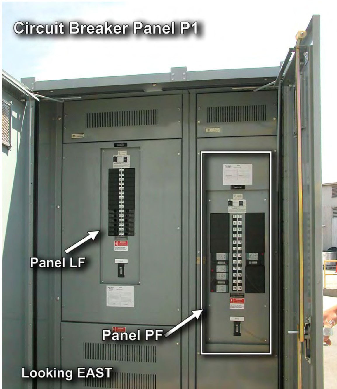
FIGURE 3b.—Circuit Breaker Panel P1. East view of opened doors showing electrical Panels LF and PF. Debris Removal System (DRS) controls are switched ONLY on Panel PF (to the right).
