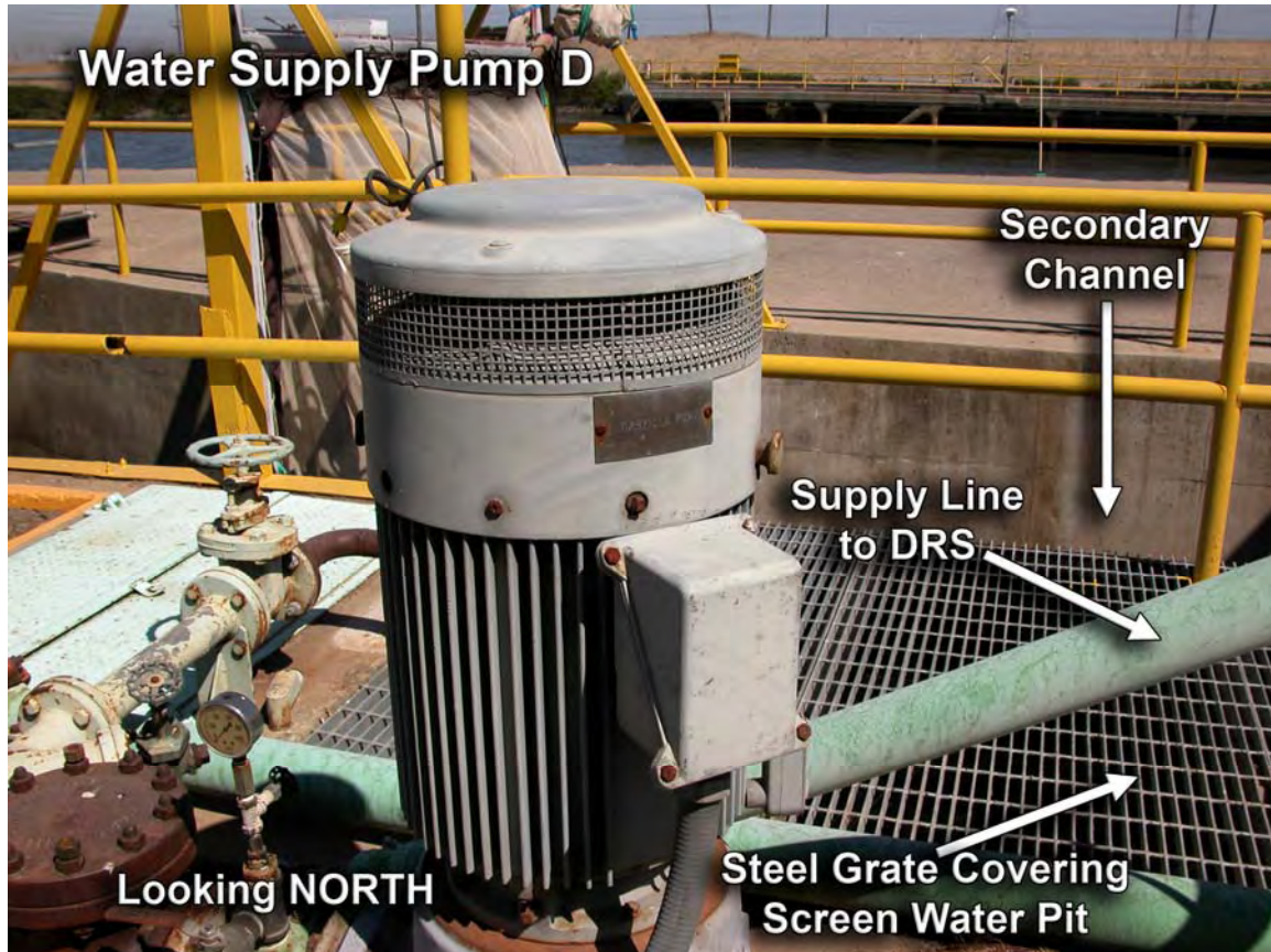
FIGURE 8.—North view of Water Supply Pump D.
