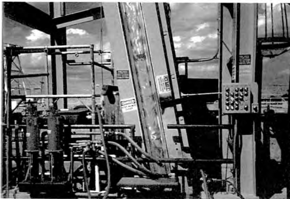
Figure 3: Close-up of spray wash filter system and control panel.
