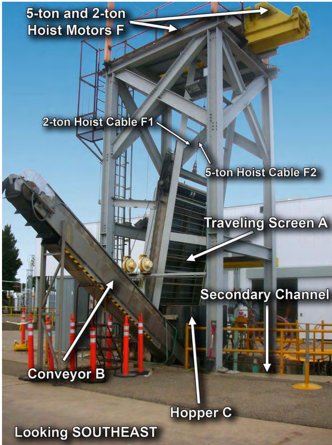
FIGURE 2a.—Southeast view of Debris Removal System (DRS). The descending side of Traveling Screen A is shown along with Hopper C and Conveyor B. The 5-ton and 2-ton Hoist Motors F are both located on the top of DRS superstructure, and 2-ton F1 and 5-ton F2 Hoist Cables are noted.
