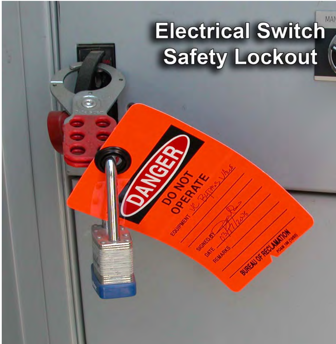
FIGURE 11.—Example Lockout/Tagout of electrical switch as found in Water Supply Pump Control Panel P3.
