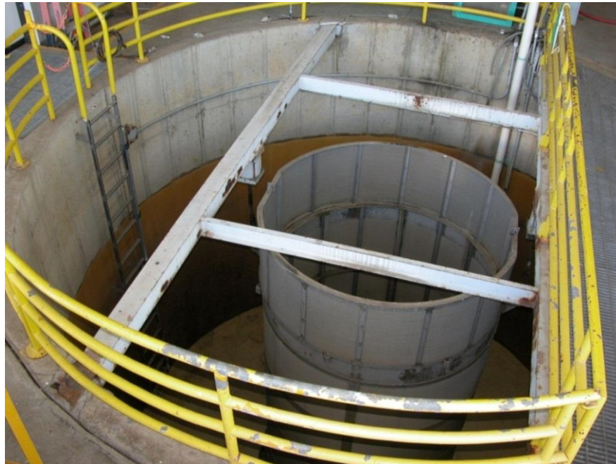
Figure 1.—Flow-through, open-end, conical-bottom, concrete holding tank at the Tracy Fish Collection Facility.
