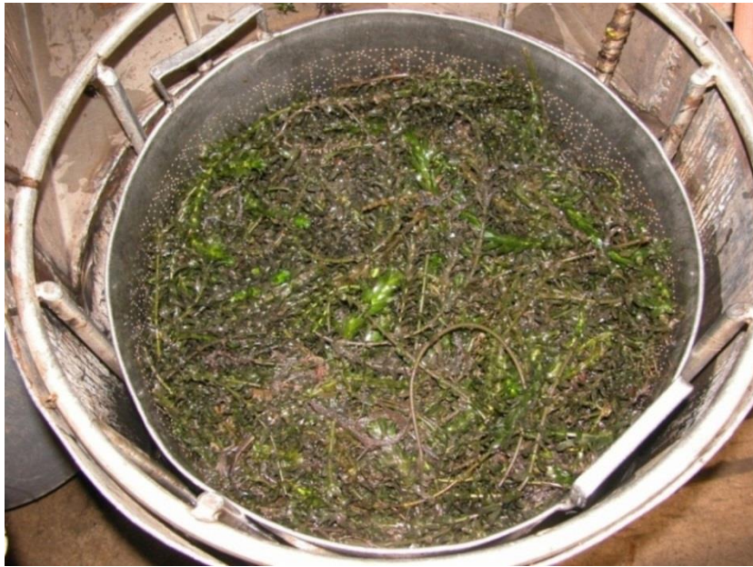
Figure 5.—Example of green debris encountered during the salvage process at the Tracy Fish Collection Facility. Green debris consisted almost entirely of Brazilian elodea during the Holding Tank Screen Lift evaluation.
