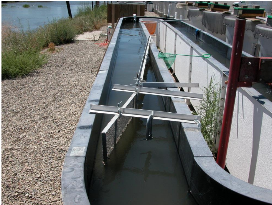
Figure 4.—Aluminum perforated plate installed across the flume at a 15 degree angle to mimic the secondary louvers and bypass.
