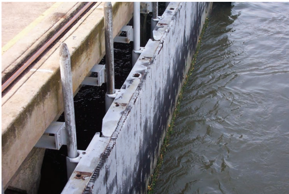
FIGURE 13.—Louver panel fouling was documented during data collection.
