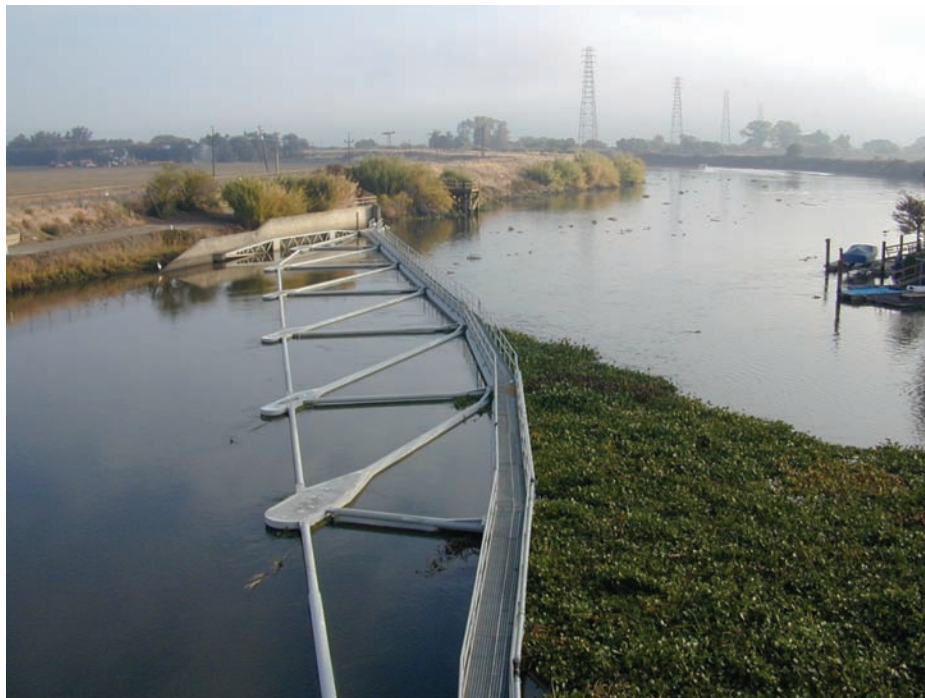
FIGURE 11.—Debris collected upstream from the debris boom. Heavy debris loads clog the facility and affect the performance of the louver system.
