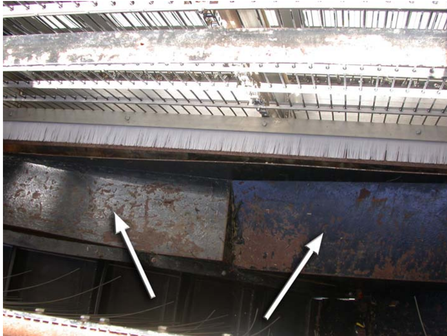
FIGURE 5a.—Before: Two, different angle, steel ledges, on the east side of the hopper (upstream side), collected much debris that the sprayers were unable to move onto the conveyor.
