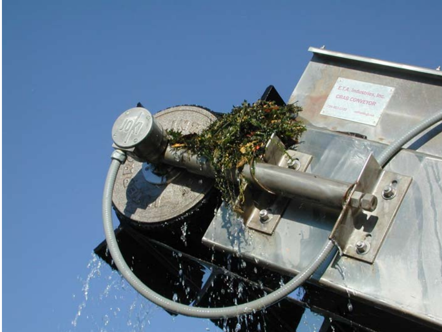
FIGURE 2a.—Before: Debris would fall off the sides of the conveyor or be blown away by the wind and therefore was not collected in the debris hauling truck.
