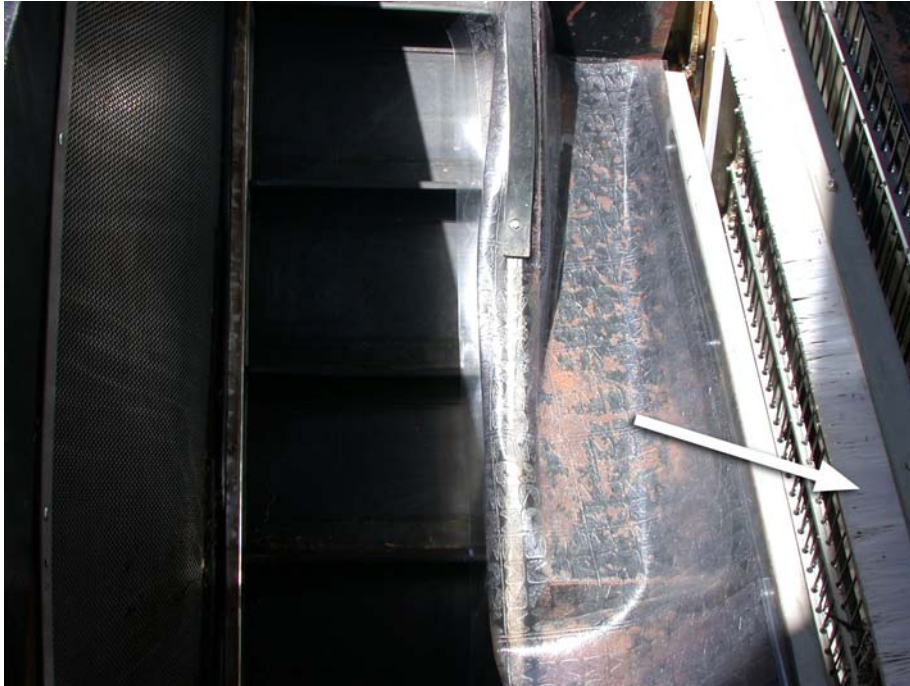
FIGURE 7.—Additional lifts were added to the traveling screen to help collect more debris.
