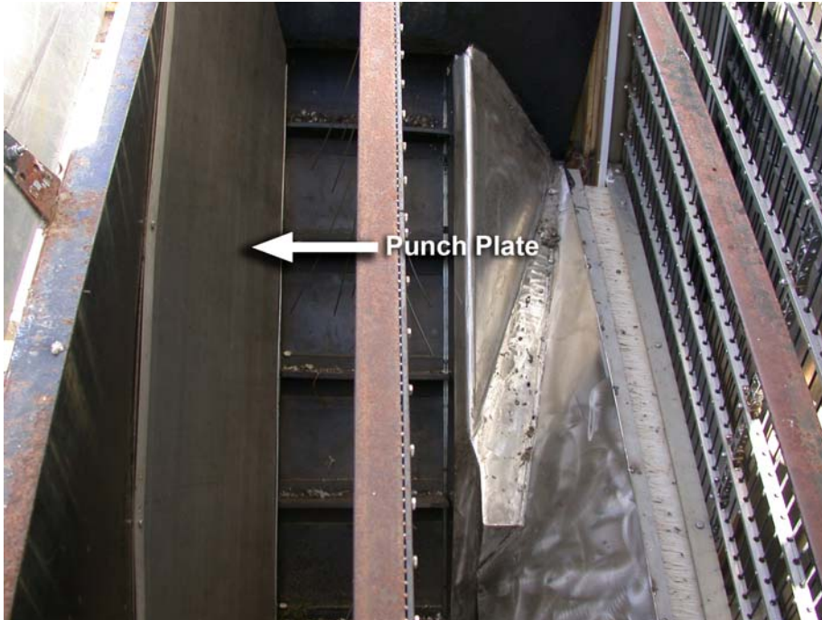
FIGURE 3b.—After: Stainless steel punch plate was installed to cover the drain tube and west gutter. This punch plate provides a slick surface, which allows most of the debris to slide onto the conveyor.
