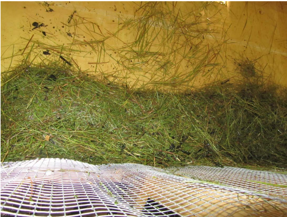
Figure A-10 - Collection of hay and woody debris in the tailbox downstream of the traveling screens
