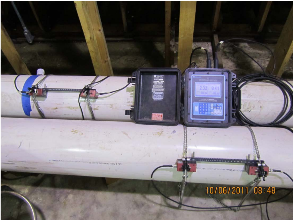
Figure A-6 - Ultrasonic flow meter on two inflow pipes (flow from right to left)
