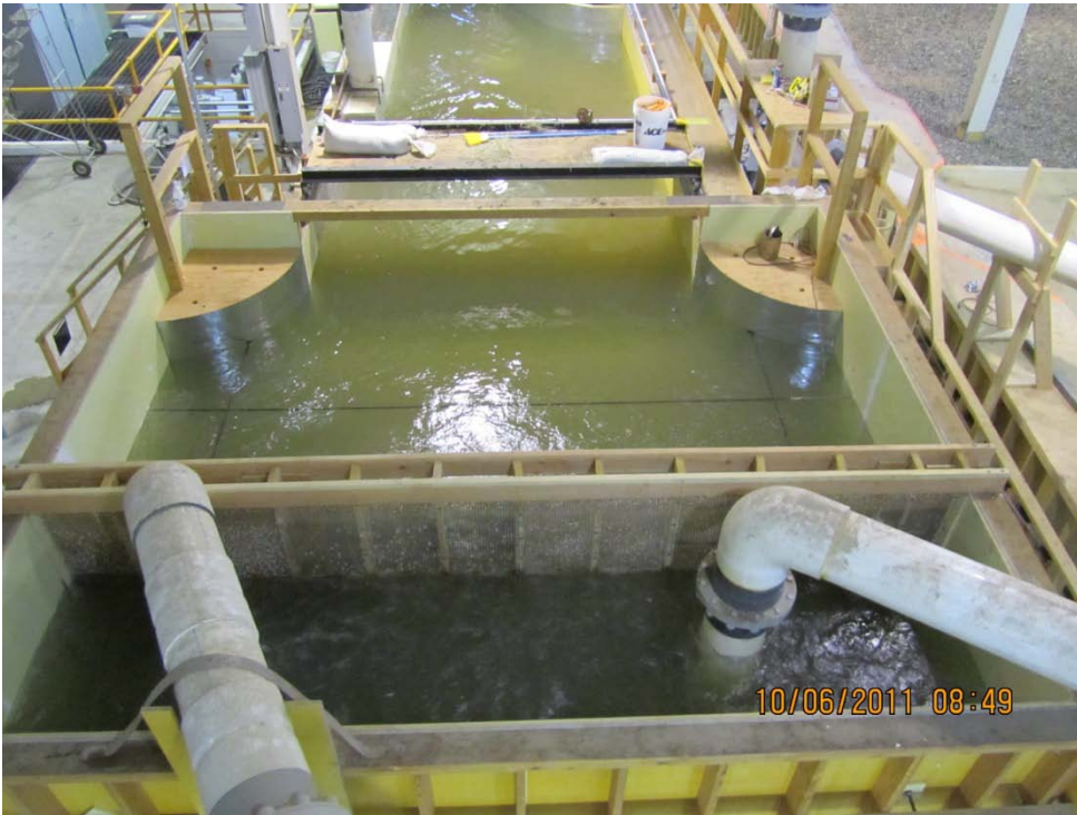
Figure A-8 - Headbox and inflow pipes 1 and 2 (flow from bottom to top)
