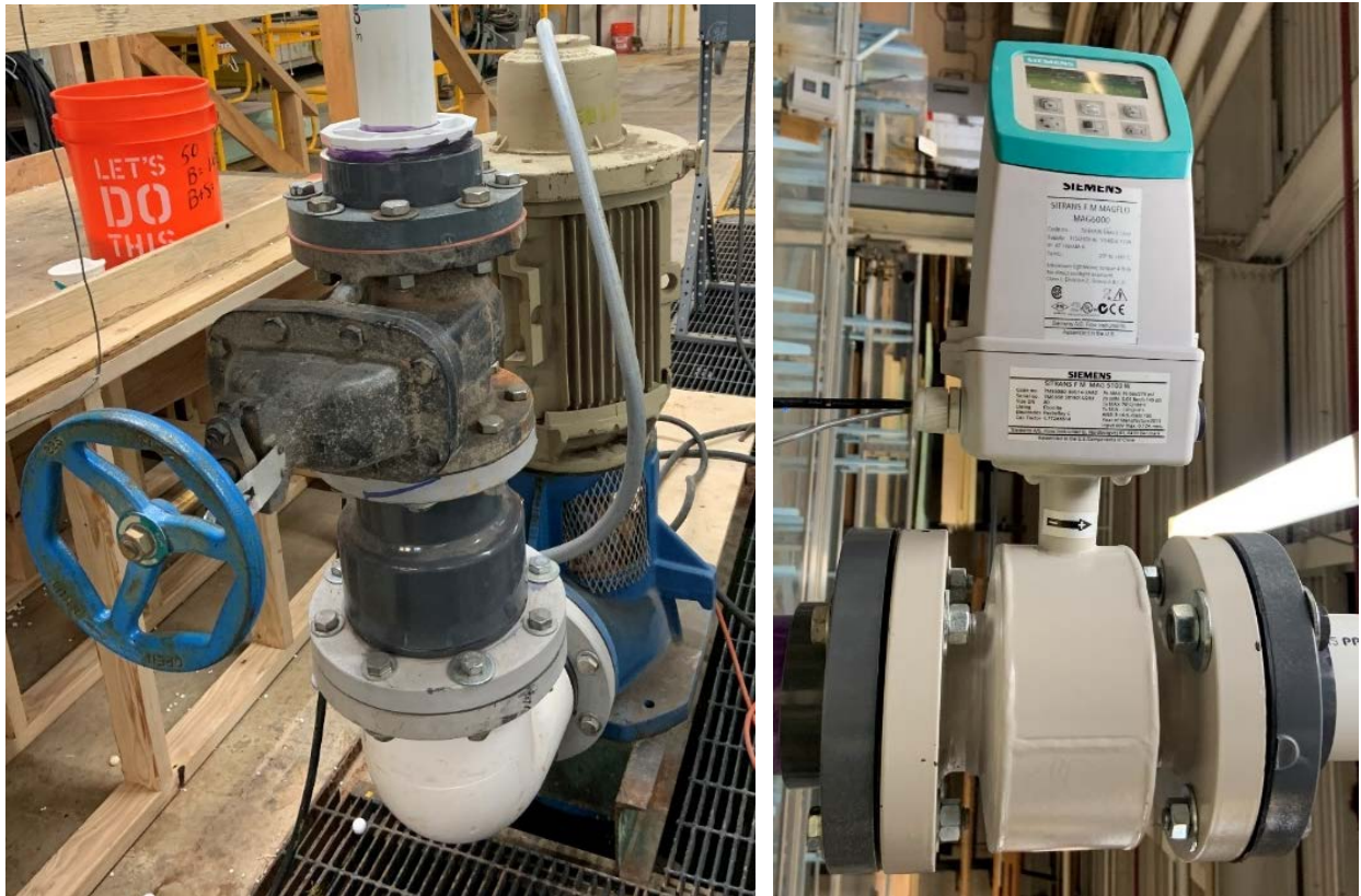
Figure 5. (Left) Vertical pump and controlling slide gate used to regulate the flow into the release pipe. (Right) Magnetic flow meter used to measure the flow entering through the auxiliary flow manifold.
