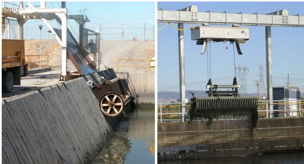
Figure 12 Trash rack cleaning at the Tracy Fish Collection Facility
