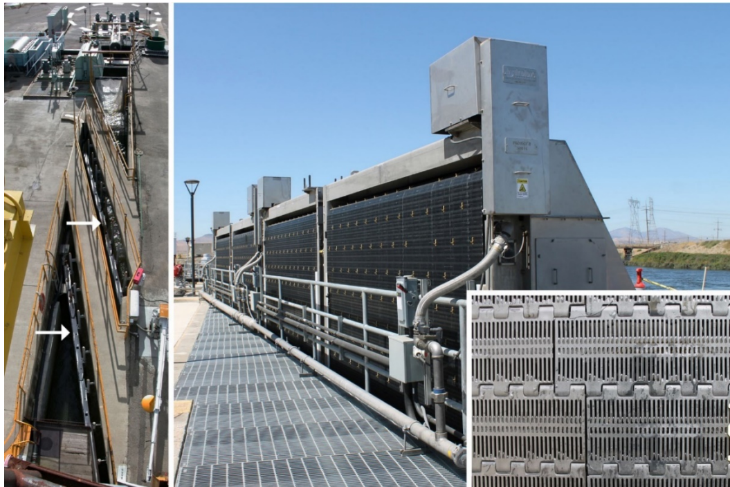
Figure 7 Secondary channel of the Tracy Fish Collection Facility
