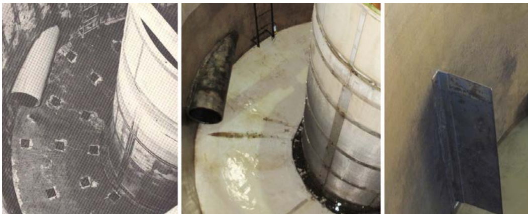
Figure 17 Holding tank at the Tracy Fish Collection Facility
