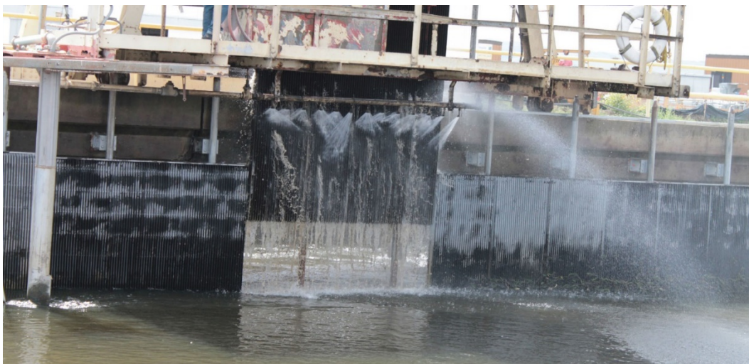
Figure 10 Primary louver panel, one of 36, lifted for cleaning at the Tracy Fish Collection Facility
