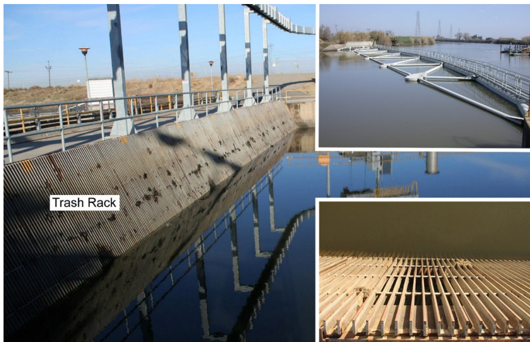
Inset: trash deflector boom (top) and view from the deck of the trash rack's vertical bars with average opening of 5.7 cm (bottom).
