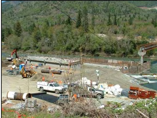
The $39.3 million Savage Rapids Dam Removal Project includes new pumping facilities and removing the dam to restore natural fish passage past the site.
