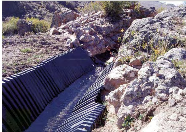
A pre-formed plastic ditch liner reduces water loss at the Pinecrest Ranch Irrigation Project.
