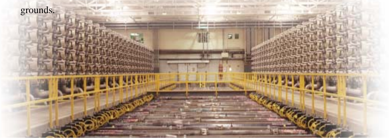
Yuma Desalting Plant Process Area
