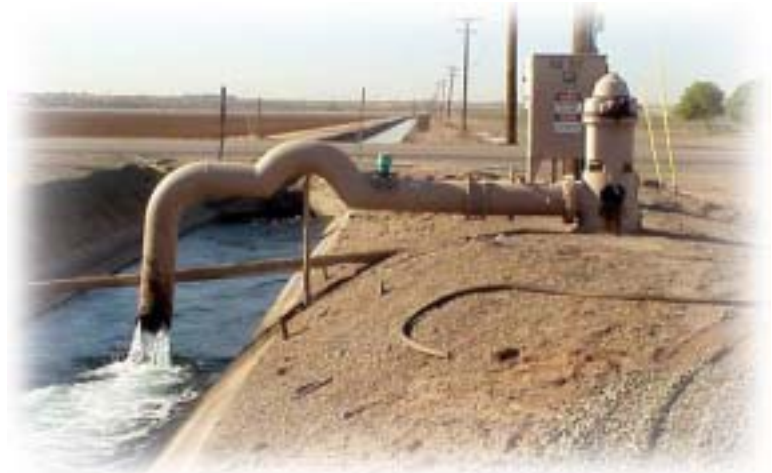
Drainage Pump Outlet Channel
