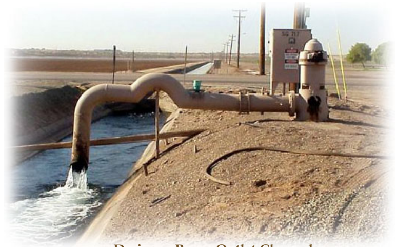
Drainage Pump Outlet Channel
