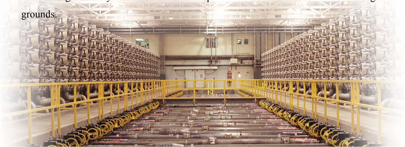
Yuma Desalting Plant Process Area
