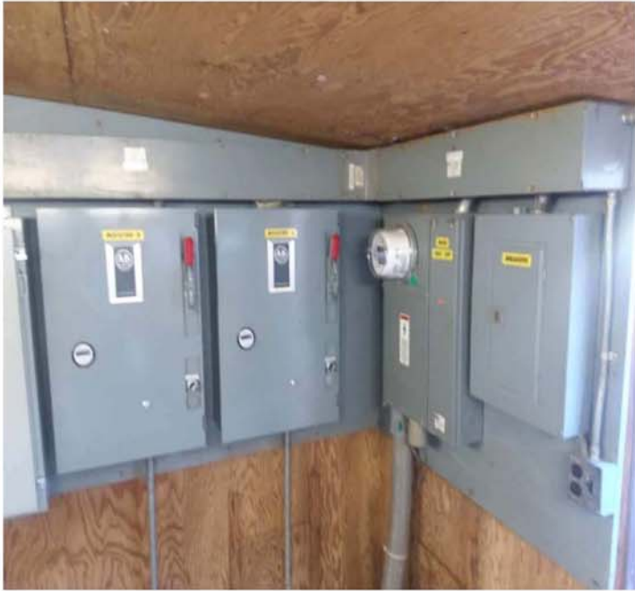
New Electrical Panels
