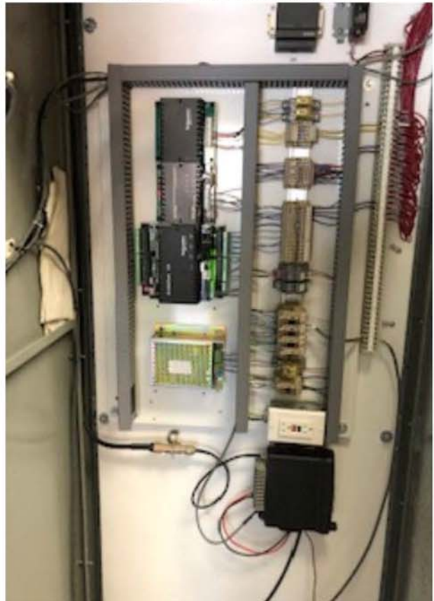
New Telemetry Panel
