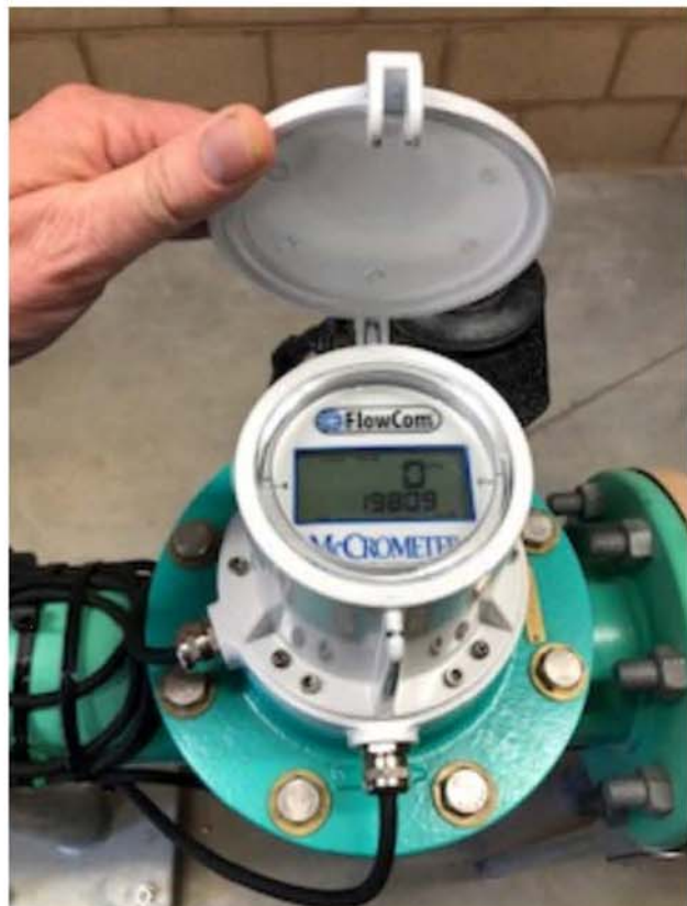
New Radio Read Well Production Meter (typical of 13)
