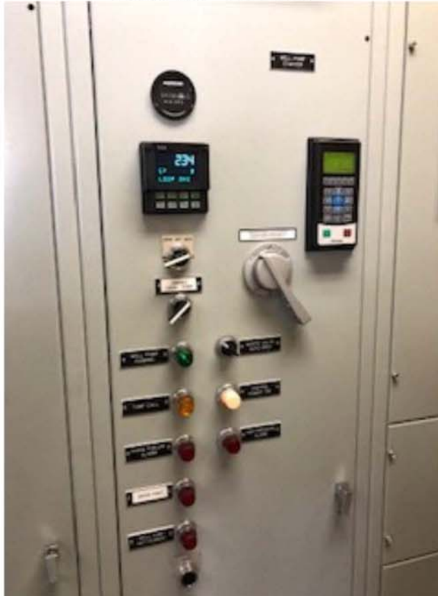
New VFD Controls
