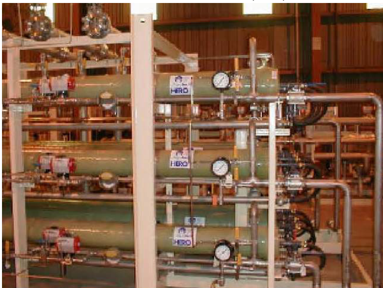
FIGURE 2.11 HIGH-EFFICIENCY REVERSE OSMOSIS (HERO) SYSTEM
