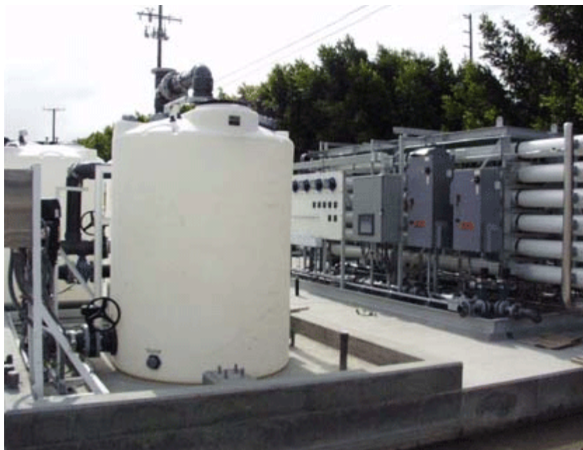
FIGURE 2.16 LBWD TWO-PASS NF PILOT PROJECT
