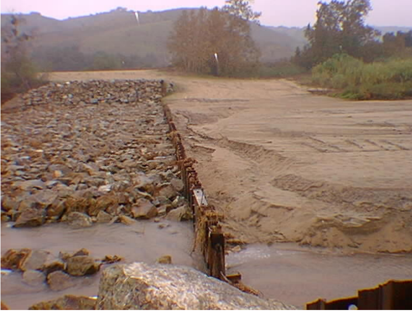
Photo 4 - Existing sheet pile dam, photo date unknown. Note the sediment accumulation in front of the dam and the riprap placed on the downstream side. The riprap extends to the right side bank.
