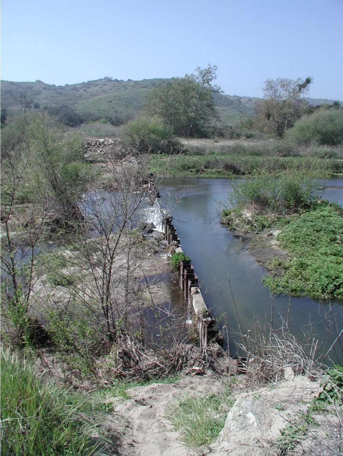
Photo 2 - Wider view of existing sheet pile dam, March 2004. Note vegetation growth and sediment accumulated in front of dam.
