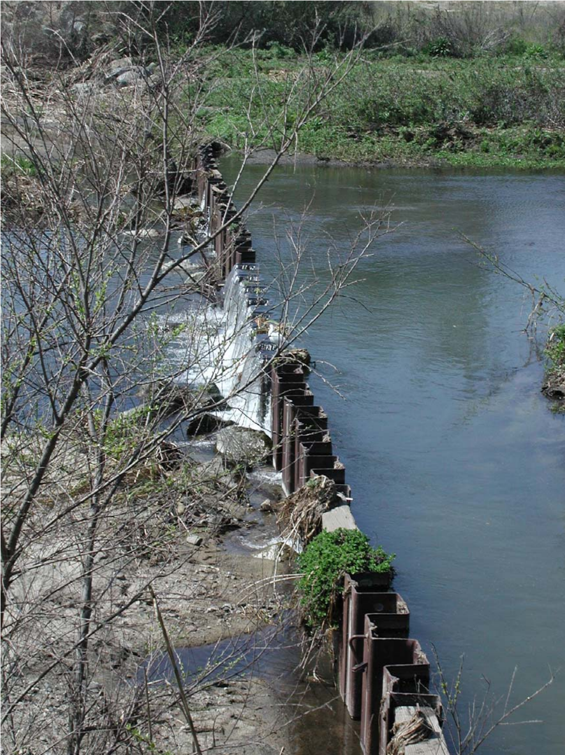
Photo 1 - Existing sheet pile dam, March 2004. Note the two stoplog slots in the lower foreground. Also note the apparent control section in the middle. The sheetpiles look to have been cut about 6" below the reported crest. Length is not measured but appears to be about 20 feet long. Note little riprap is seen.
