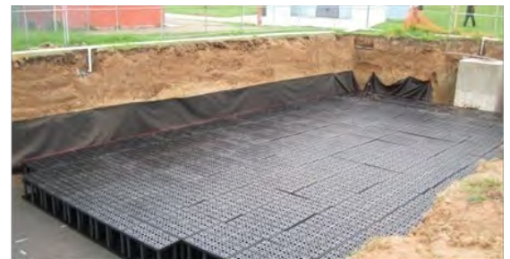
Subsurface Infiltration Basin
