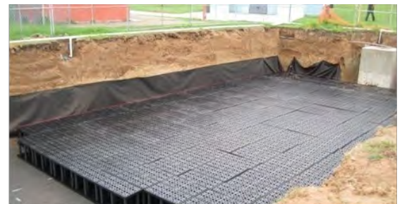
Subsurface Infiltration Basin
