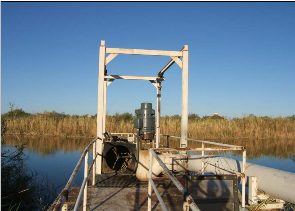
Figure 6. Irrigation pump and location of screen samples deployed at Martinez Lake inlet canal, Imperial National Wildlife Refuge.
