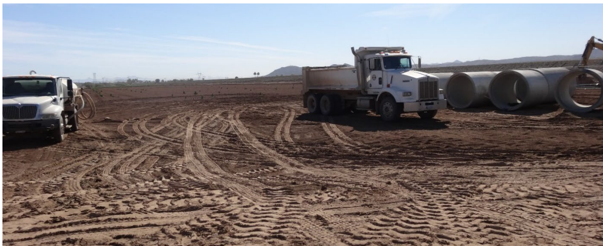
Figure 16 Photo of a Fallowed Field Being Used as a Staging Area for the Five Gates Reconstruction Project (credit: B. Barker, May 25, 2021).
