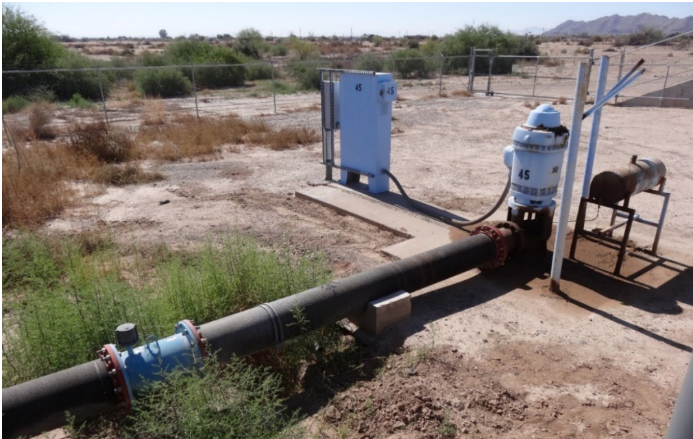
Figure 5 Photo of an Irrigation Supply Well for the Pima Canal with a Flow Meter Installed in the Discharge Pipe (Credit: B. Barker, May 24, 2021).
