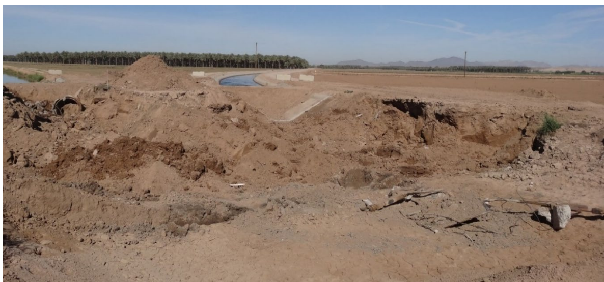
Figure 15 Photo of Five Gates Reconstruction Project in the Bard Water District (credit: B. Barker, May 25, 2021).
