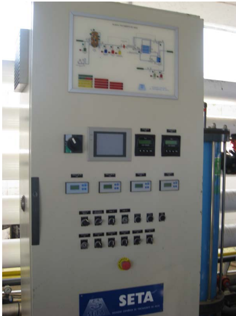
Figure 2-6: Seawater RO Pilot Plant
