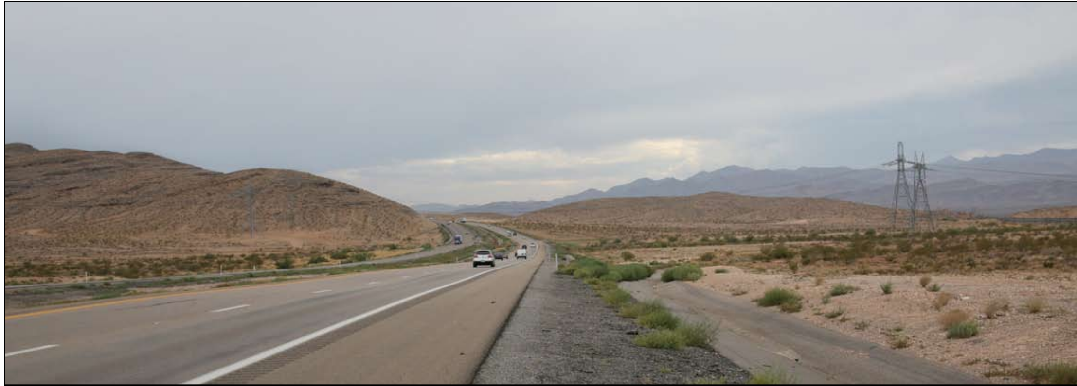
Existing Condition - Existing IPP 500kV lattice structure transmission line and the existing Crystal-McCullough 500kV lattice structure transmission line crossing Interstate 15
