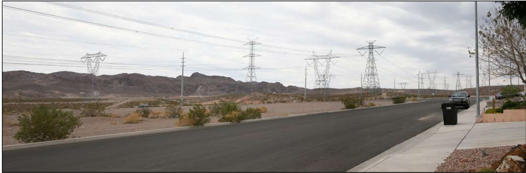
Simulated Condition - Proposed Southern Nevada Intertie Project single-circuit 500kV steel lattice structure transmission line
