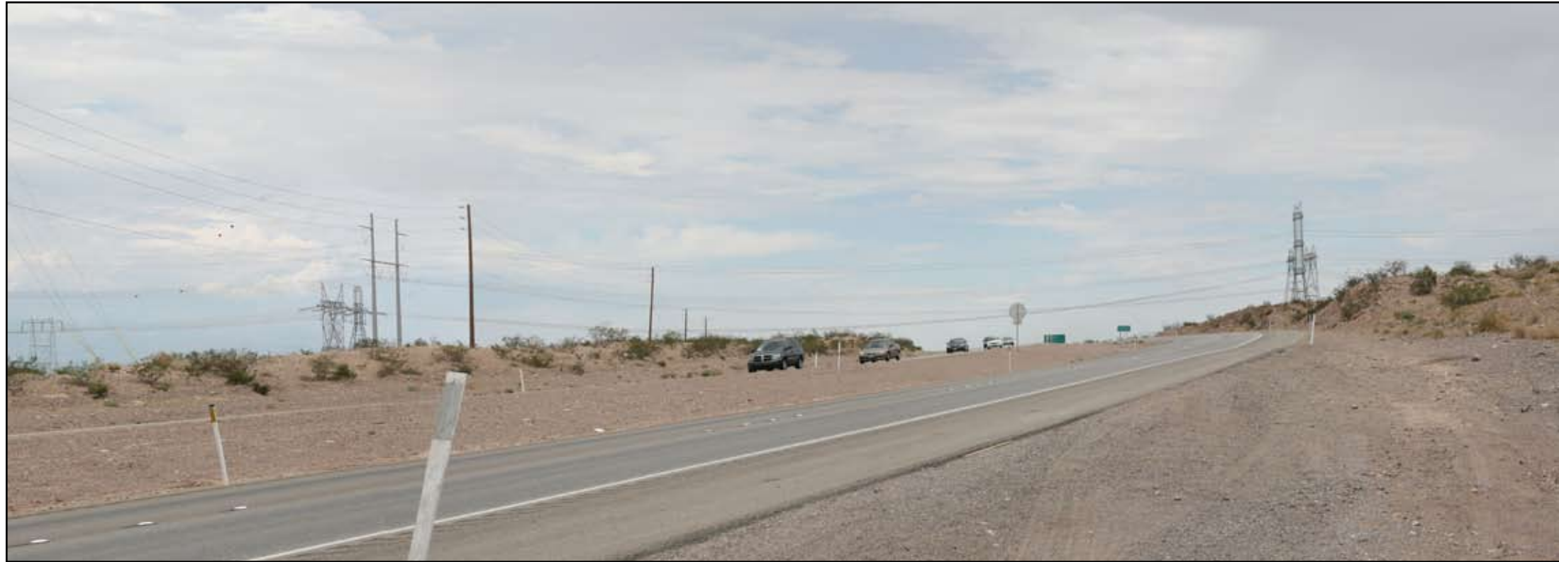
Existing Condition - Existing IPP 500kV lattice structure transmission line, existing Crystal-McCullough 500kV transmission line and existing Harry Allen to Mead double-circuit, 500kV transmission line crossing Highway 93/95
