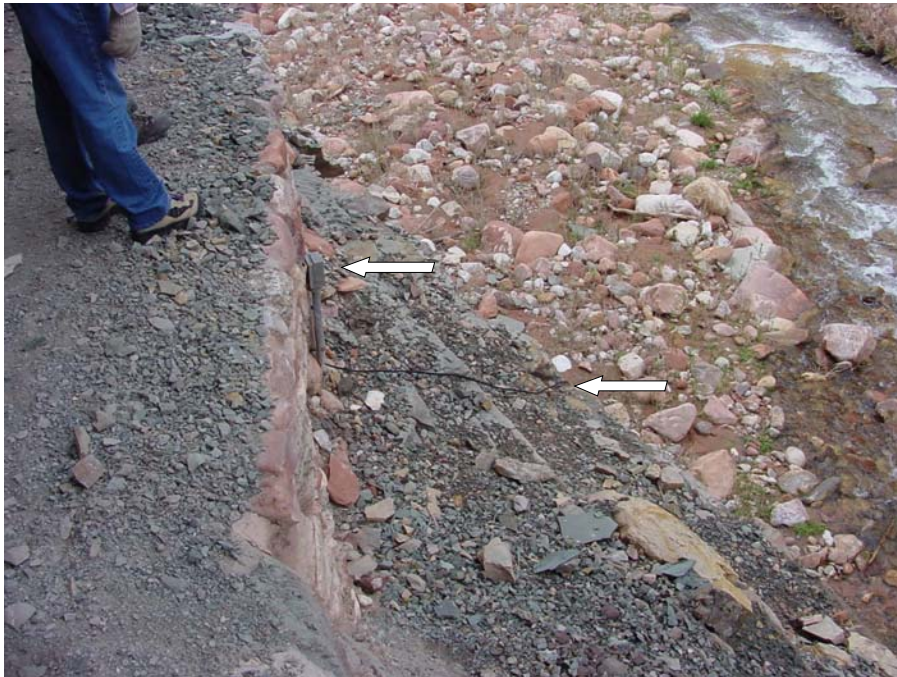
Figure 4. Test station at pipeline station 563+03. The test station (top arrow) is of a different design and materials than the original cathodic protection system materials. The test station does not have a rheostat or shunt and appears to connect an anode to the pipeline. The anode cable is exposed between test station and lower arrow, and is susceptible to damage.
