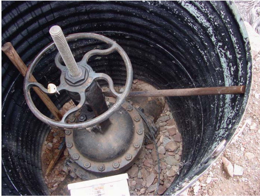
Figure 1. Typical valve box. Cast iron valve is electrically isolated from aluminum pipeline by insulated flange kits on each side of the valve. Cables are attached to the pipeline flanges and terminate in insulator bonding box (lower portion of figure). Isolation of the valve from the pipeline results in the aluminum pipeline being divided into electrically isolated sections.
