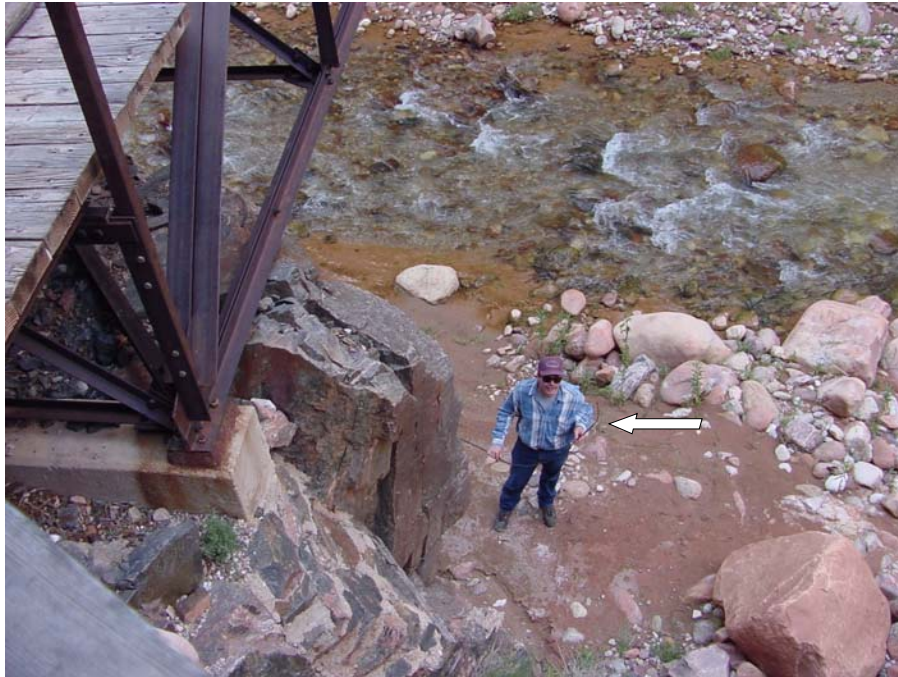
Figure 3. Anode 7 at pipeline stationing 242+30. Anode cable has been severed (arrow) and appeared to have been severed for some time. It is speculated that the anode cable was severed by the buildup of debris on the cables during flash flooding.
