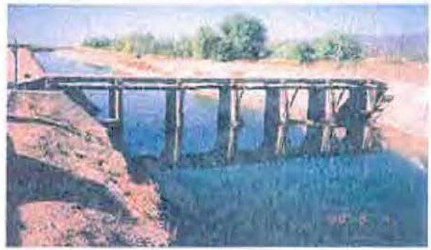
Turnout #6 checkboard structure.
