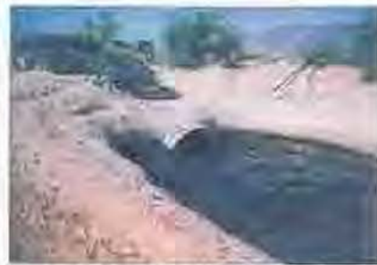
Figure 3-14 CMP culvert for Turnout #8.
