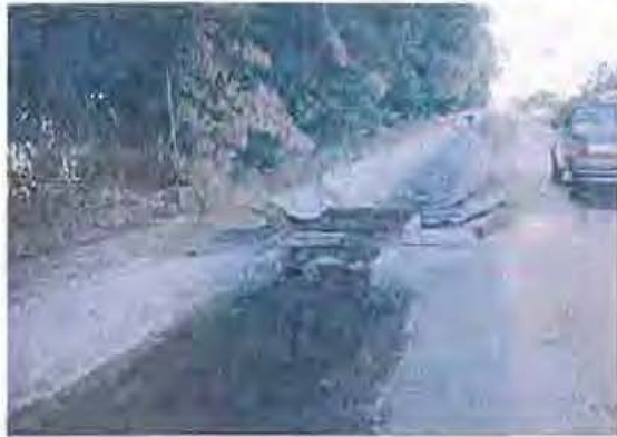
Turnout #13.5 checkboard structure.
