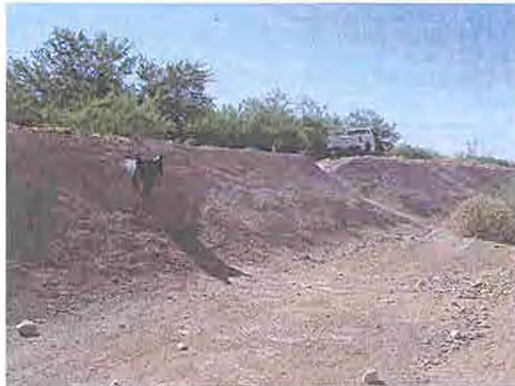
Photo 14 24 inches CM pipe with flap valve at the east side of the Canal. Behind the truck, concrete lined waterway into the Canal from the road. Note that the Canal is silted and mounded with dirt and tumble weed. There are many low points of road along the way to the Cowtown Bridge to drain some sheet runoff.
