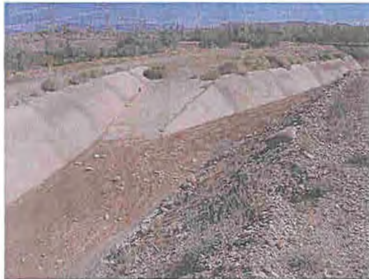
Photo 20 At 2.9 miles, looking northwesterly at the access ramp to the upstream direction. Canal is silted with mud and loose rocks from the east side bank
