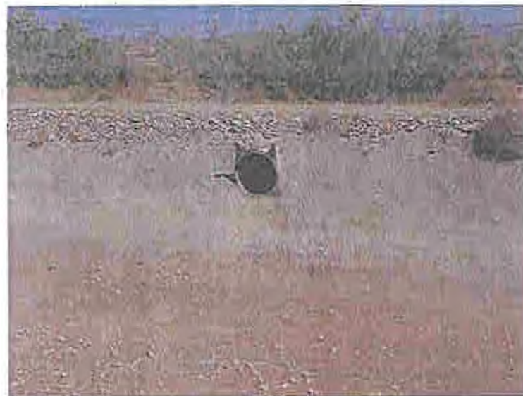
Photo 26 At 4.5 miles, looking westerly at 24 inches pipe into the Canal with flap valve removed. Canal is silted.
