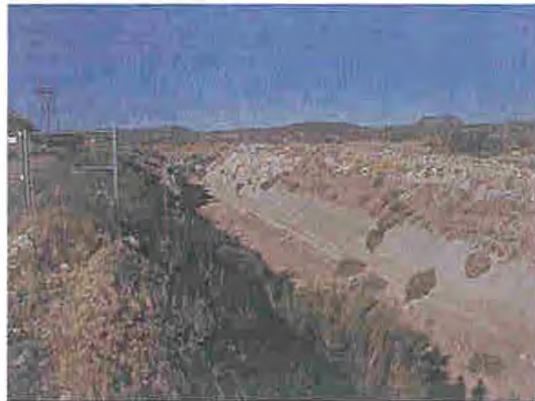
Photo 2 At just downstream of the diversion works, Canal silted with falling dirt from the west bank, looking downstream
