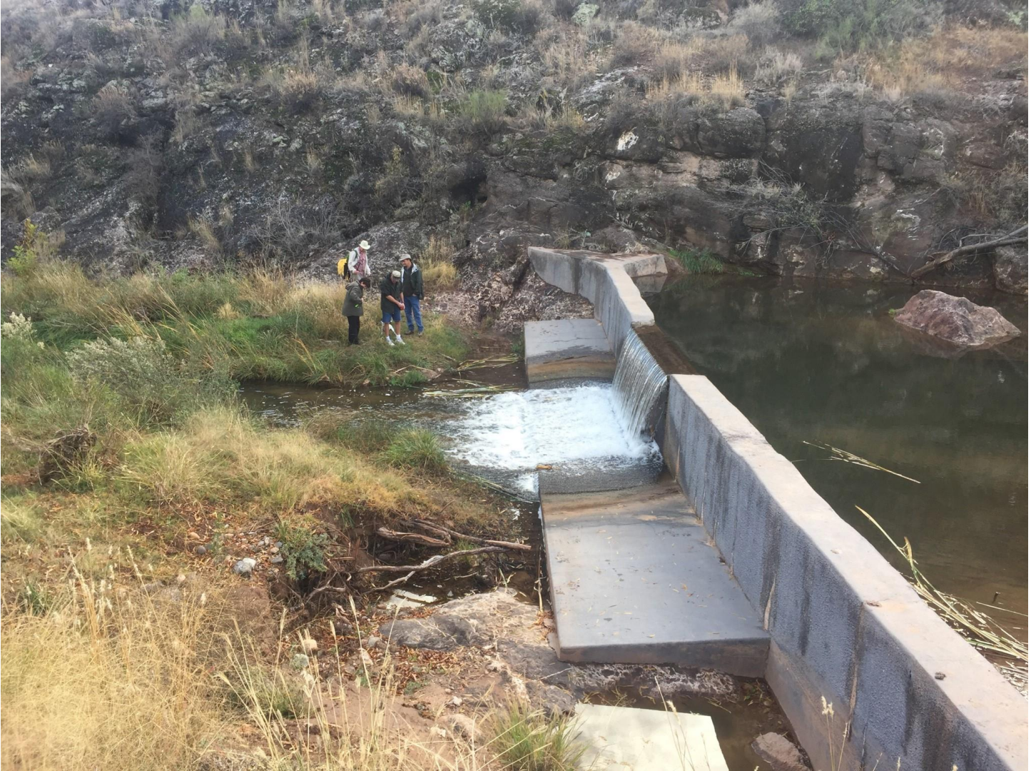
Figure 7. Spring Creek fish barrier.
