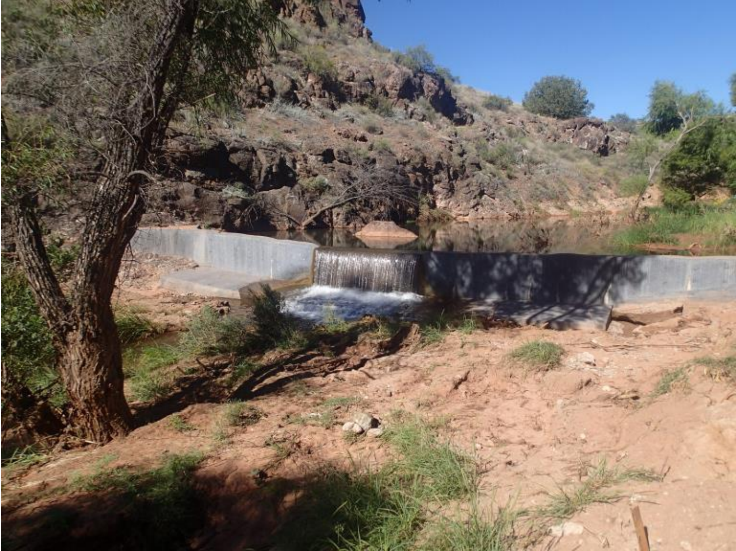
Figure 8. Spring Creek fish barrier.
