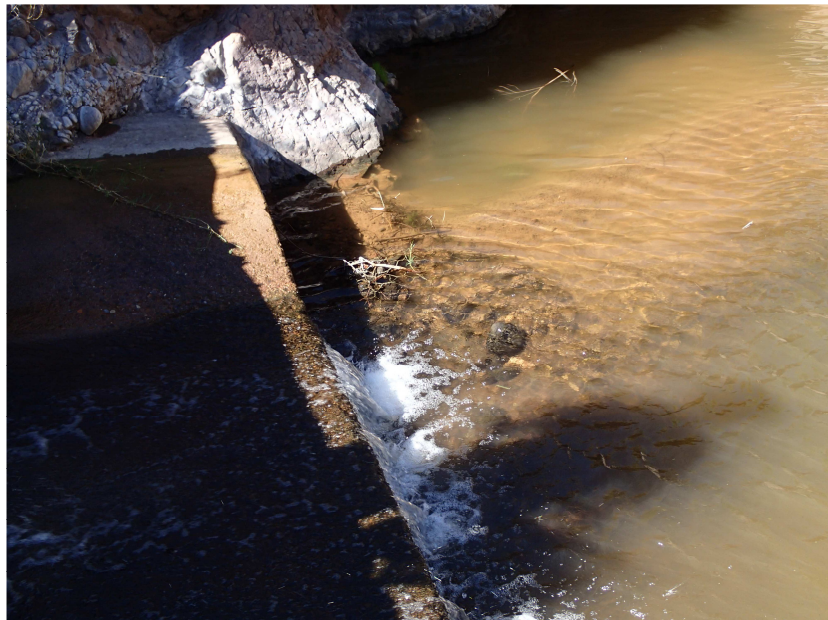
Fig. 2. Hot Springs Canyon, Cochise Co., Arizona, showing exposed wire gabion at the base of the constructed fish barrier apron on river left; October 16, 2014.
