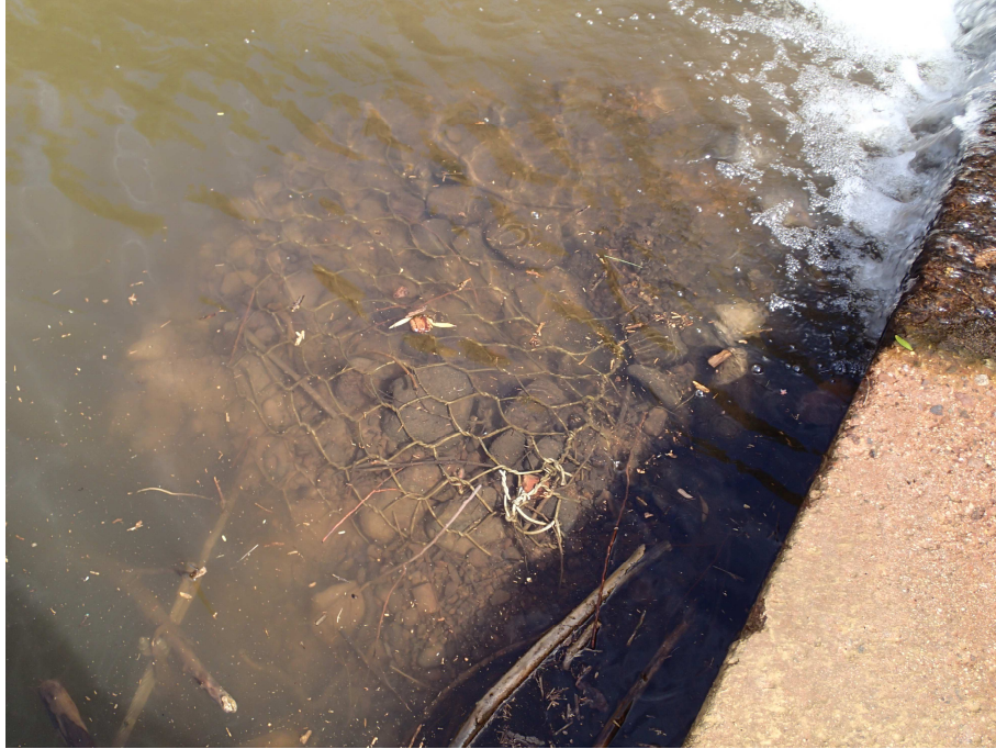
Fig. 4. Hot Springs Canyon, Cochise Co., Arizona, showing exposed wire gabion at the base of the constructed fish barrier apron on river left; October 28, 2013.
