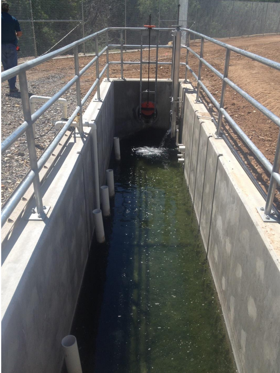
Figure C: ZZ Sump, located on the southeast, downstream area of the facility.
