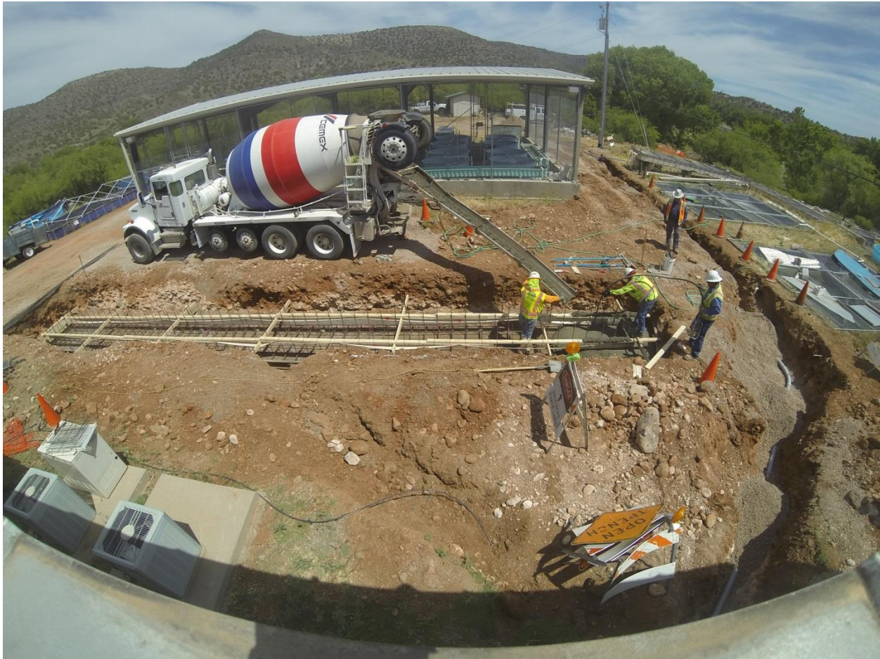
Figure A: Pouring concrete for the central trough of the Phase 1 raceways. Old ponds and tanks can be seen on the right side of the picture.
