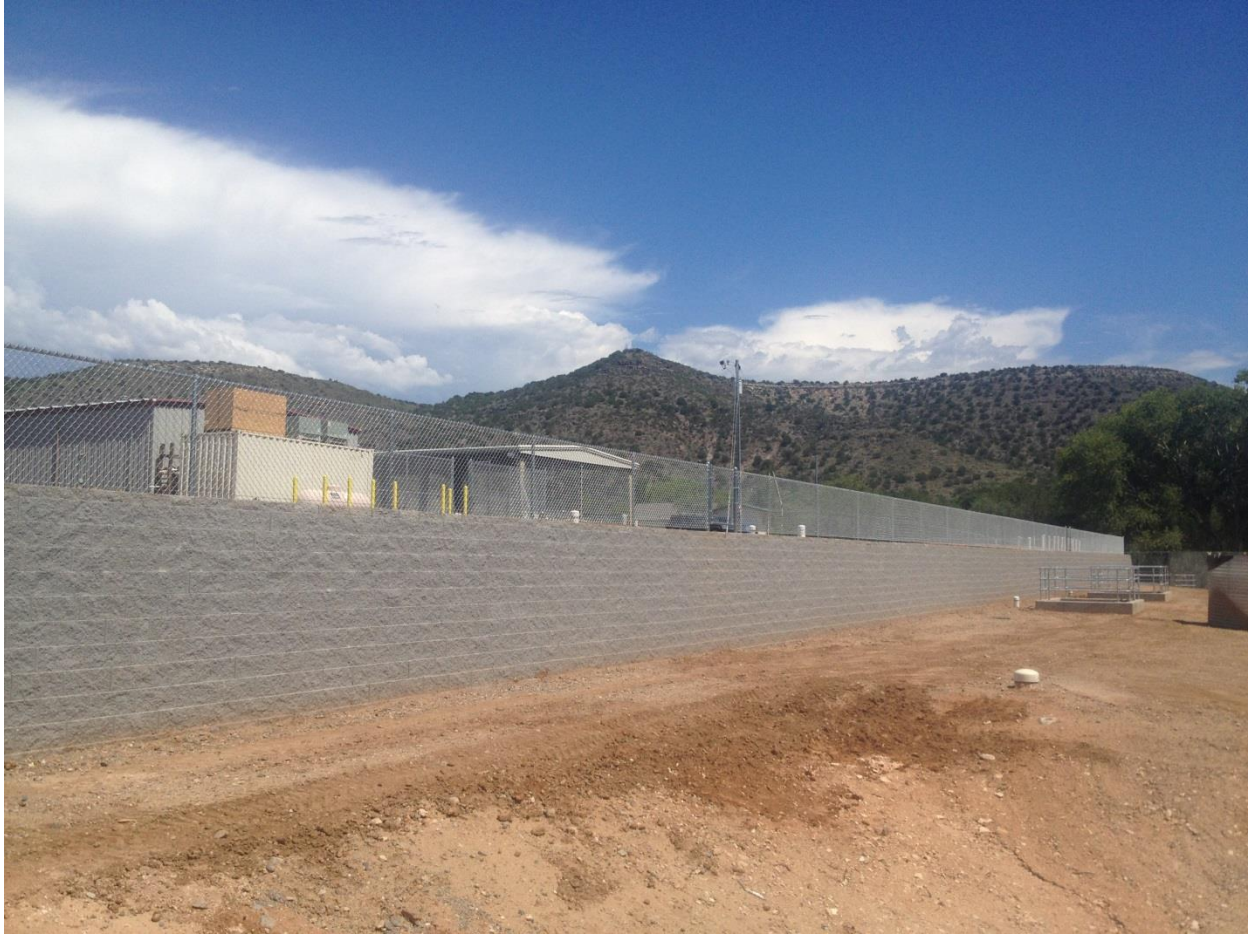
Figure E: Completed Phase 2 retaining wall. Collection sumps for the lined ponds are shown on the right side of the picture.
