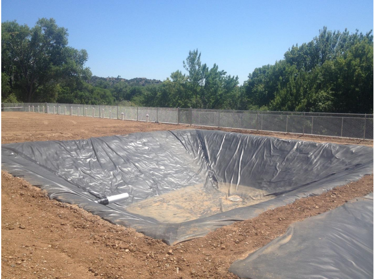
Figure D: Lined pond with 30,000 gallon capacity installed on the upper tier created by the Phase 2 retaining wall.
