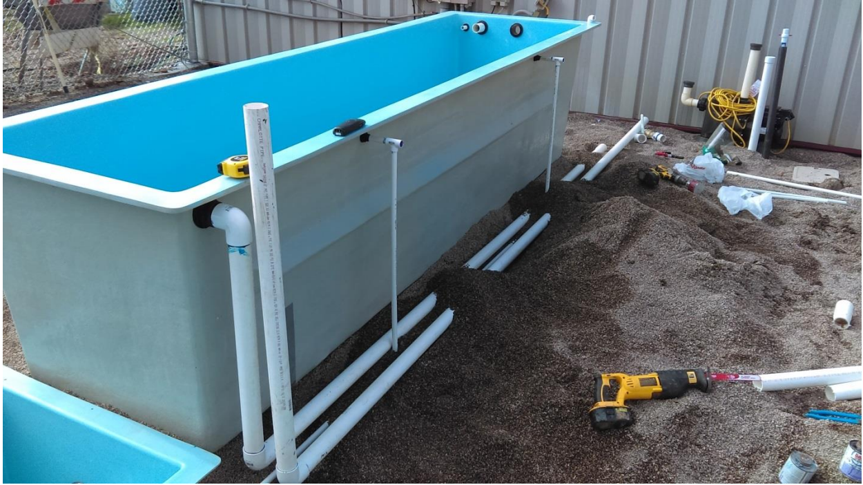
Figure B: Plumbing of new Phase 1 raceway, with collection sump on left.
