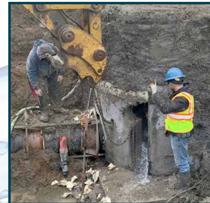
Chris Haines, P.E. Civil Engineer for Rural Water Division, Dakotas Area Office, works with a contractor to disassemble a valve vault at a Mni Wiconi repair location. (Reclamation photo)
