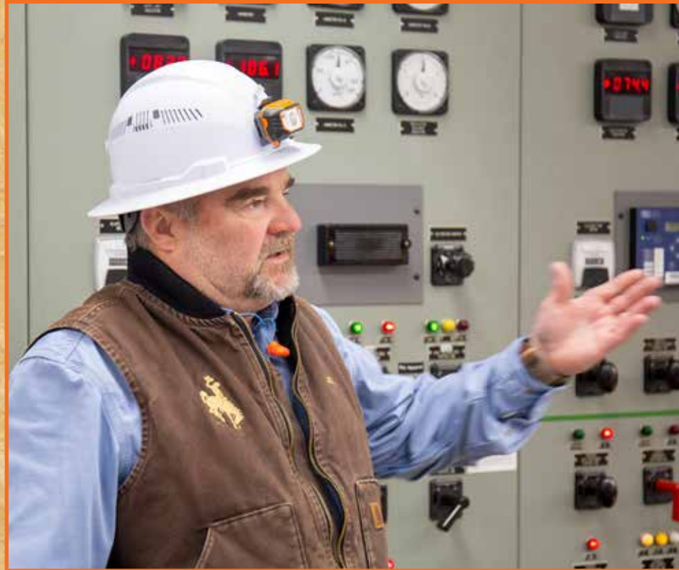
Left: Buffalo Bill Powerplant Supervisor Jack Buffkin explains how power is generated to volunteer members of the visitor's center at Buffalo Bill Dam and Shoshone Project Complex outside of Cody, Wyoming.
