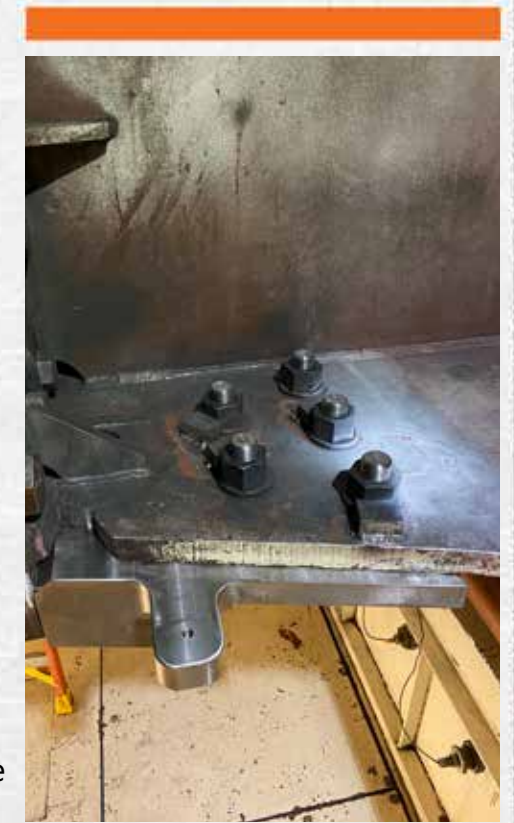
Top view of the rotor spider arm with the interim repair bracket installed.
